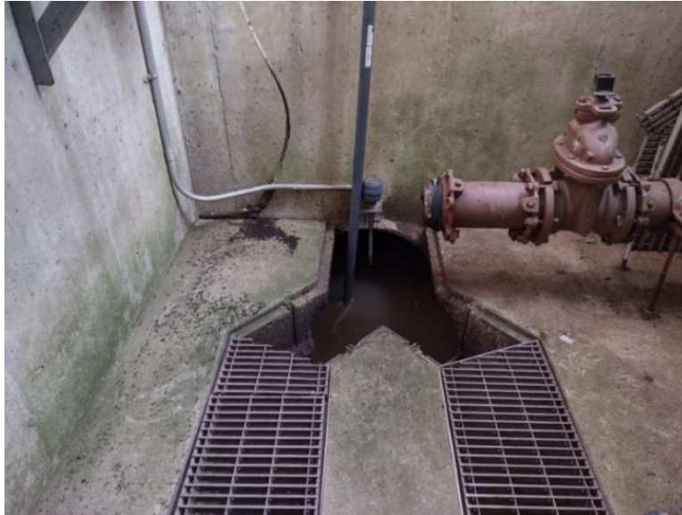
Figure C-1: Photo of UVAS continuous monitoring probe installation location in the Fleetwood WWTF influent trough from November 30 th , 2023, through January 19 th , 2024.
