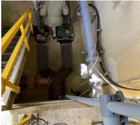
Figure 1: Photo of UVAS continuous monitoring probe installation location in the Fleetwood WWTF influent trough
