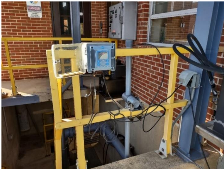
Figure C-2: Photo of HACH SC200 controller and UVAS continuous monitoring probe mounting installation location in the Fleetwood WWTF primary treatment from November 30 th , 2023, through January 19 th , 2024.
