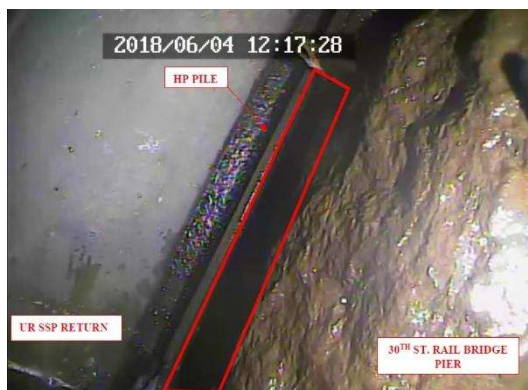
The above photograph was taken of a gap in the bulkhead on the upriver side of the SEPTA Rail Bridge before work commenced.
