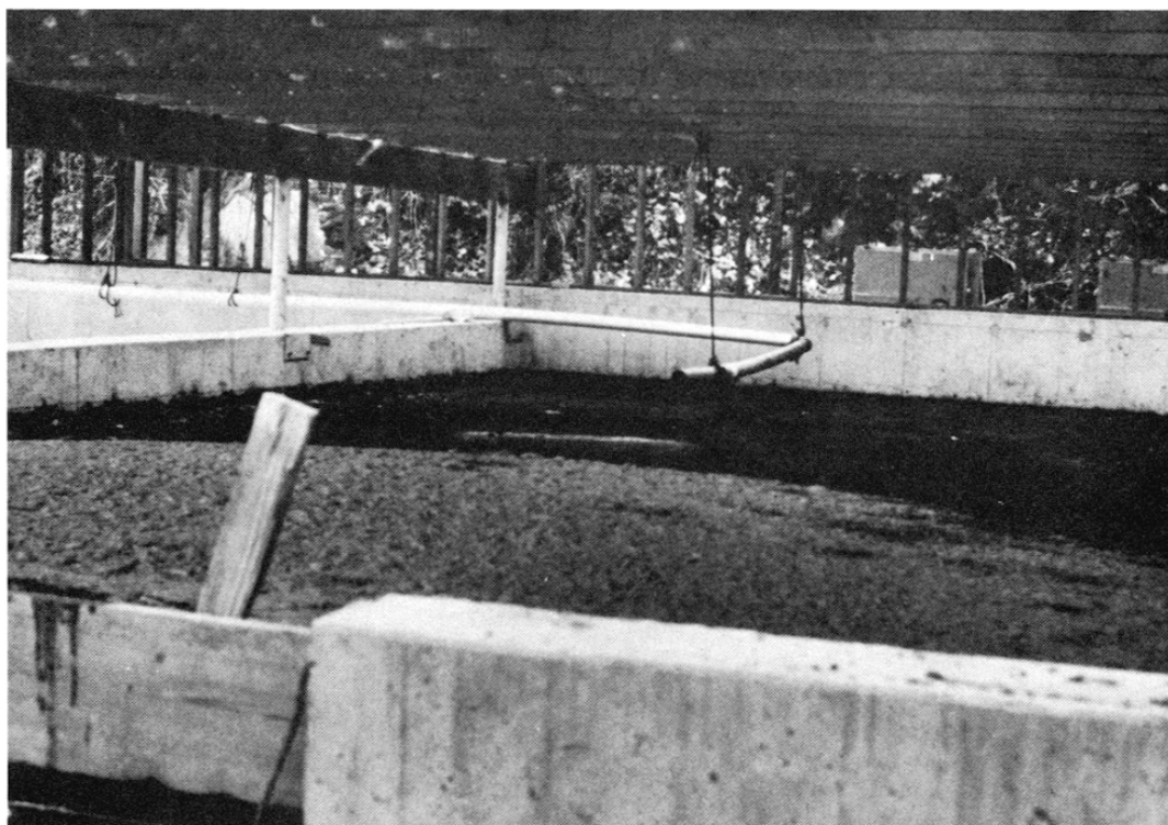
Figure 2.5 Processing of Waste Activated Sludge 5
