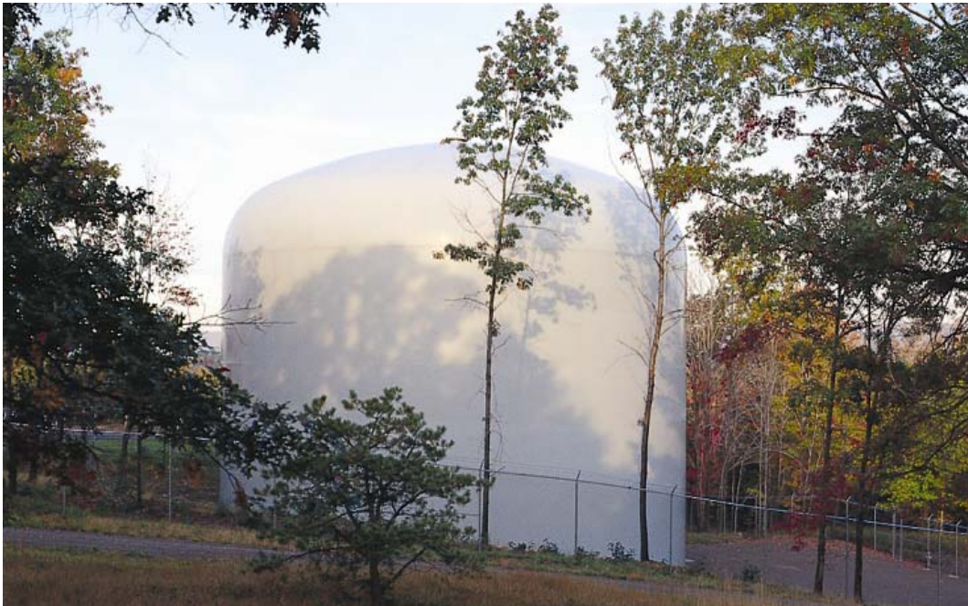
Figure 3.2 – Ground Level Tank
