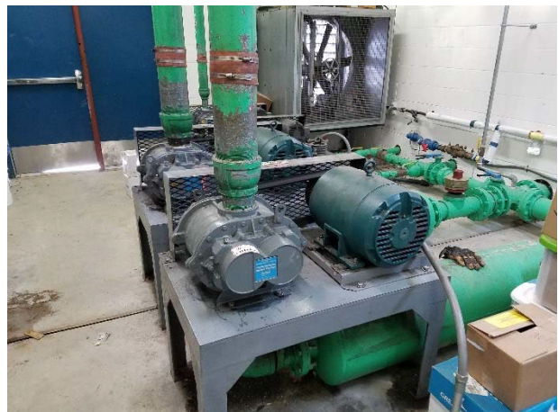
Aeration Rotary Lobe Blower System
