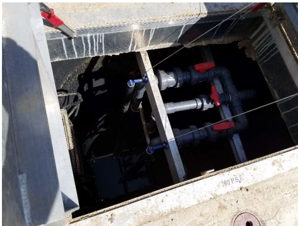
Wet Well for RAS Submersibles
