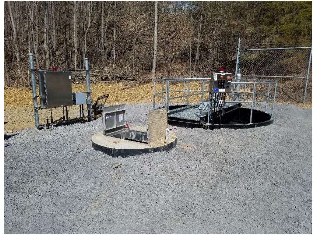
14'-diameter Secondary Clarifier & RAS Pit
