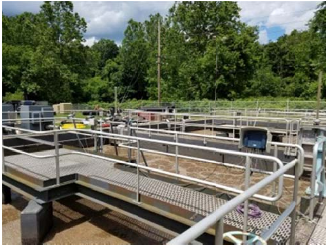
Photo 1: Aeration Probes & Controller at Tank 2
