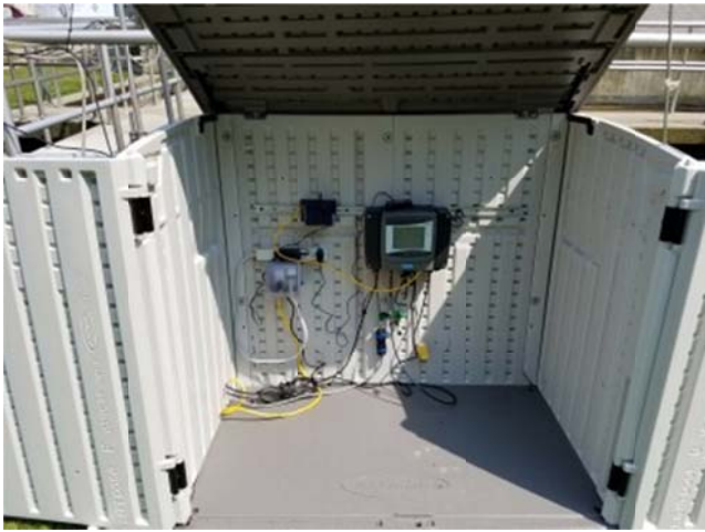
Photo 7: Remote SCADA II
