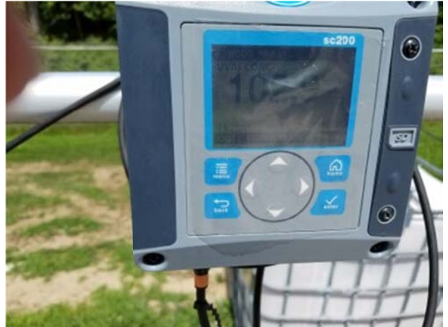
Photo 4: Controller for BOD Probe
