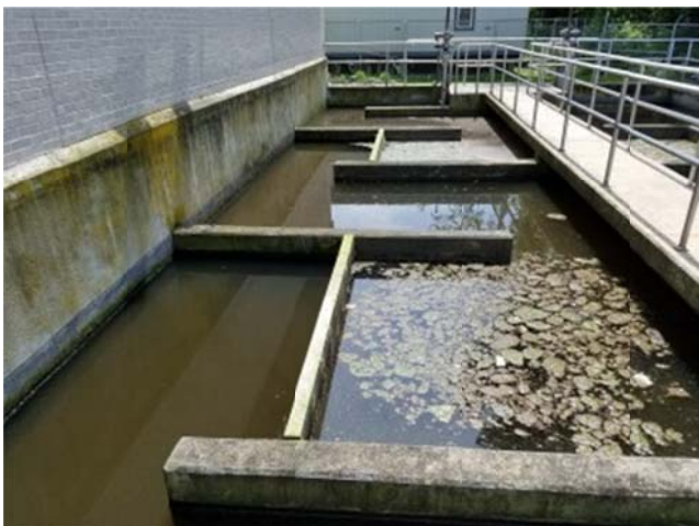
Photo 11: Chlorine Contact Tank w/ TSS
