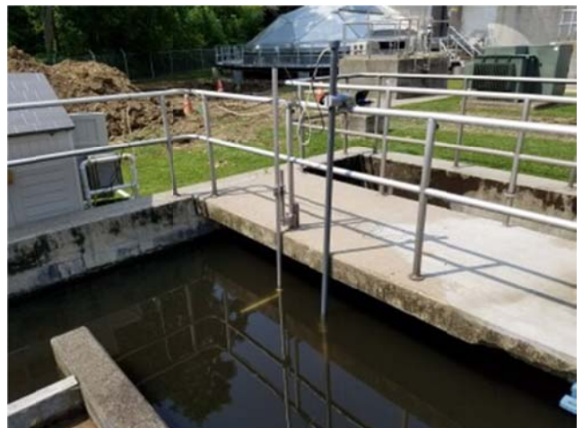
Photo 6: Effluent Probes in Cl 2 Contact Effluent End
