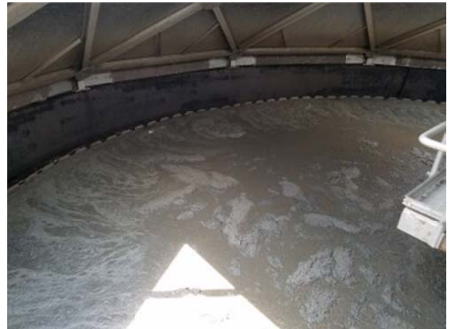
Photo 18: Sludge Thickener insettleability
