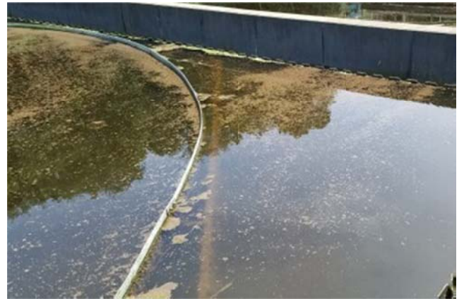
Photo 14: Denitrification in Secondary Clarifier
