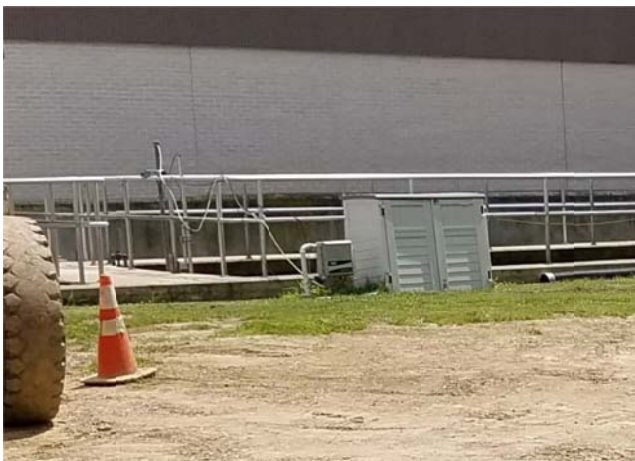
Photo 5: Chlorine Contact Tank with NO 3 , NH 4 Probes
