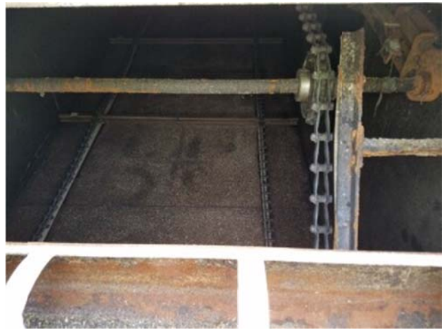
Photo 20: Spalling inside Primary Clarifier
