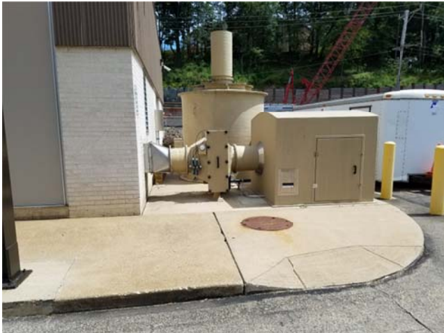
Photo 21: New Activated Carbon Air Filtration System
