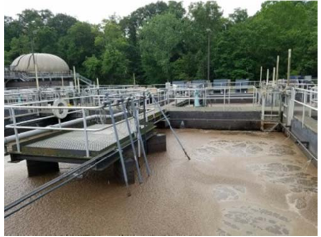
Photo 2: Aeration Probes in Tank 5
