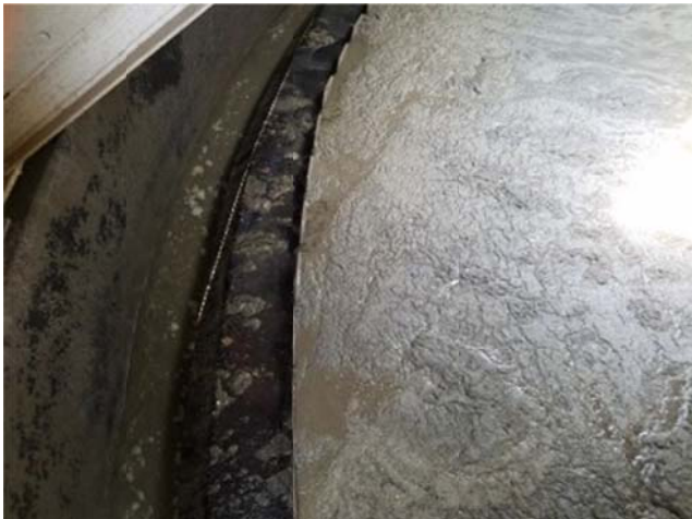
Photo 17: Rising solids / carryover in sludge thickener
