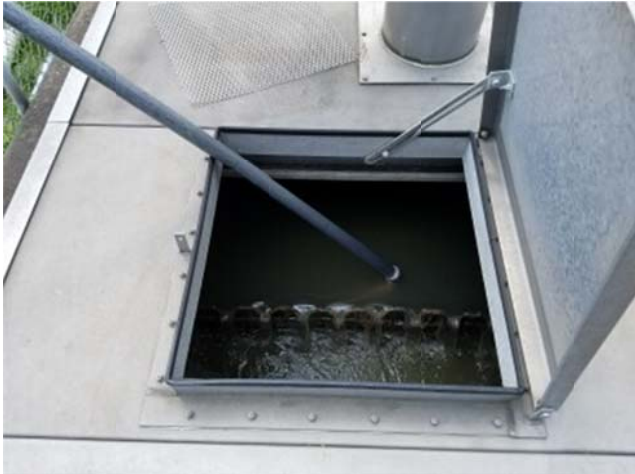
Photo 3: BOD probe in Primary Clarifier effluent
