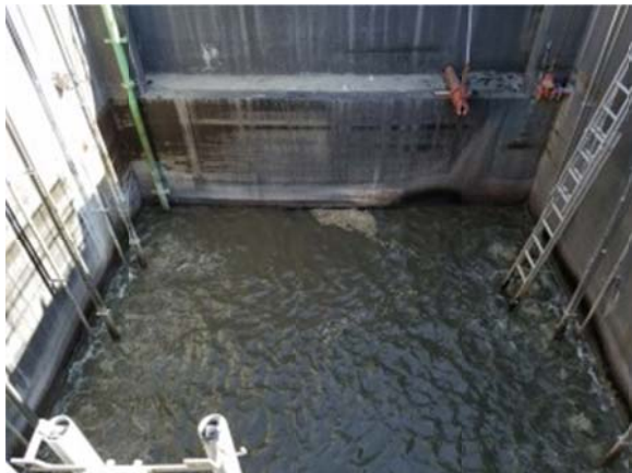
Photo 9: Raw WW Equalization Tank
