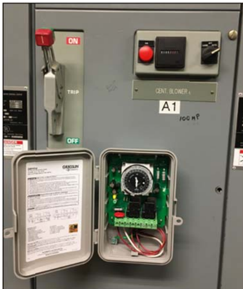
Photo 11: Power Logging at Main Blower Controls (note new timer box on blower motor starter's door)
