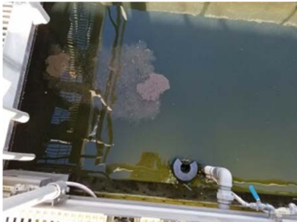
Photo 7: Denitrifying Solids in Clarifier
