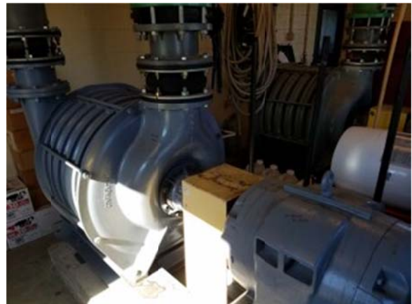
Photo 10: Main Aeration Centrifugal Blower
