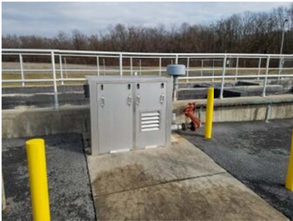
Photo 17: 7.5 h.p. Blower for Effluent Freshening
