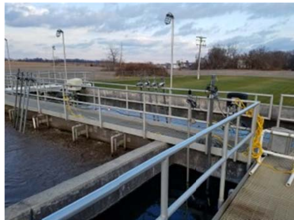
Photo 4: Immersion probes in Train 1, both stages
