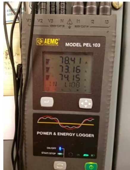
Photo 12: Amperage reading for running blower motor
