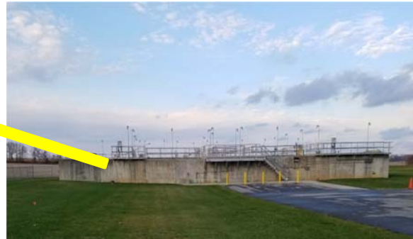
Photo 2: 2-Stage Sequox Package Plant, 2 trains
