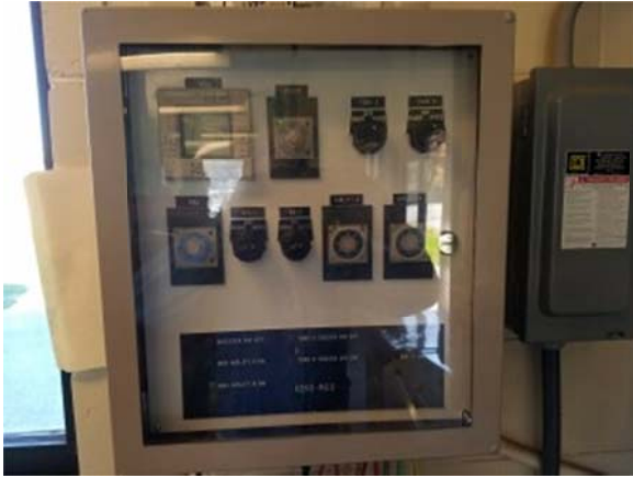
Photo 13: Sequox Control Panel
