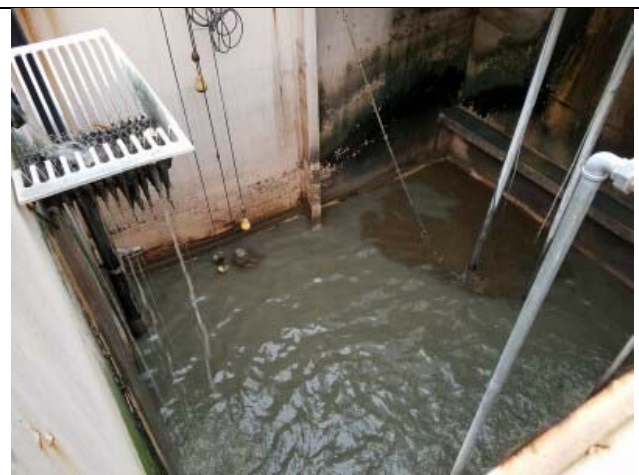
Alleged Paint Dumping (balled oil paint in corner)
