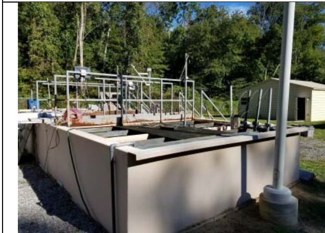
Probe Assembly at B-Side
