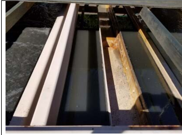
Photo: Grey Water of Clarifier Effluent
