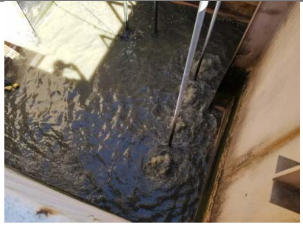
Photo: Surge Tank—Septage and Low Level
