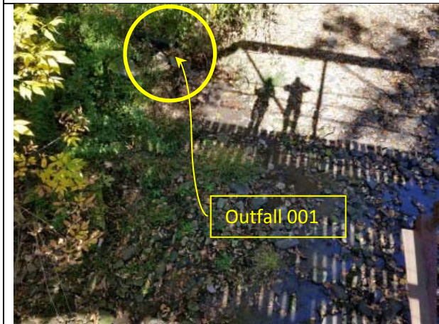
Unlabeled Outfall Pipe / Grey Discharge
