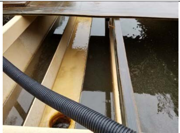
MLSS Carryover in Clarifier Trough
