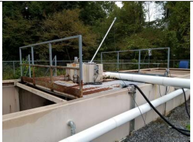
UVAS Placement at Inflow Splitter
