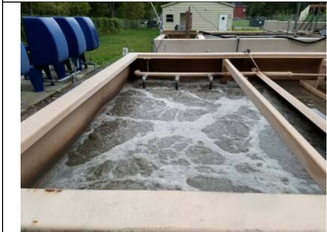
A-Side Under Aeration
