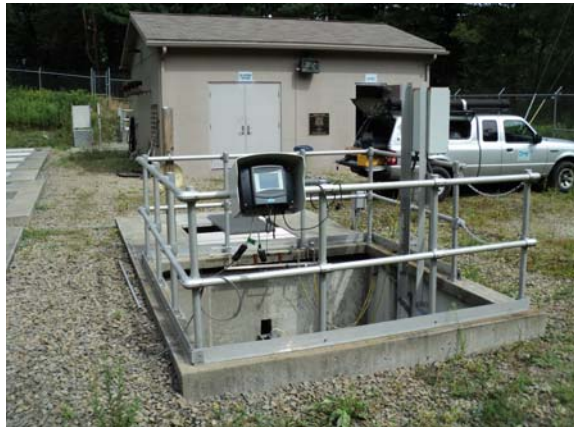
Figure F.3: SC1000 display at post aeration tank
