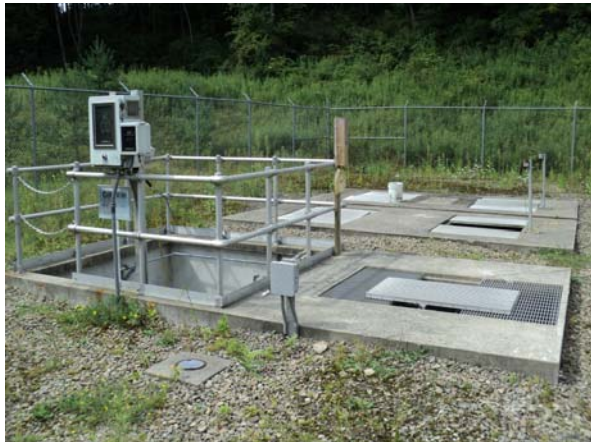
Figure F.5: Sludge holding tanks, post settling, post aeration
