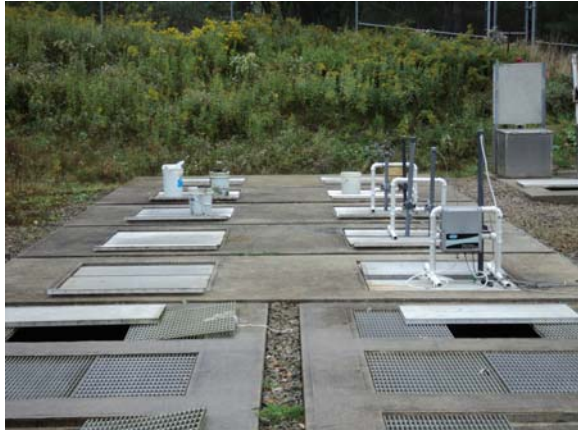
Figure F.1: On-line monitoring probes in aeration tanks
