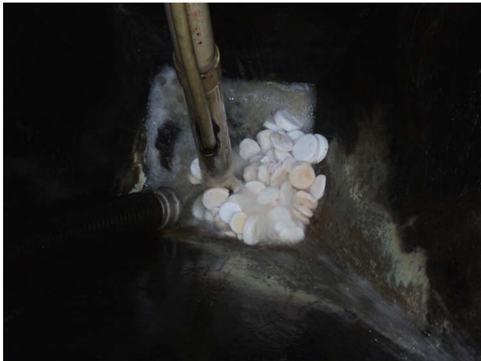
Figure F.8: Accumulation of chlorine tablets at the bottom of the post settling tank
