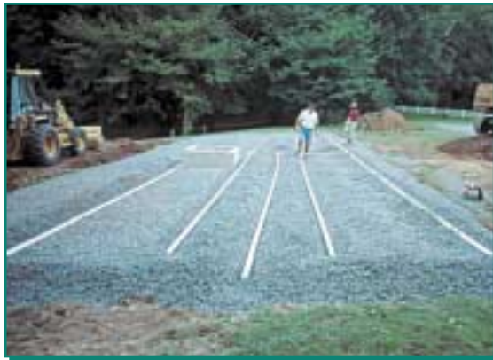
At-grade bed with distribution piping
