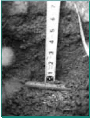
▲ 15. Tubing emitting wastewater
