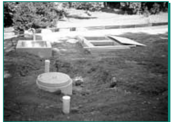
Septic, rock, and sand filter tanks
