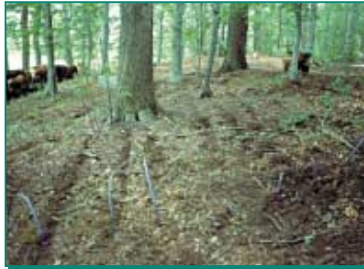
Ends of installed drip tubing
