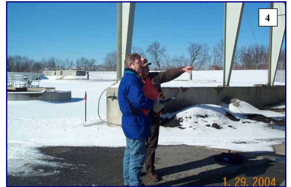
Dewatered Sludge Storage Pad – Non-potable Water Spigot May Serve For Wetting Yard Waste
