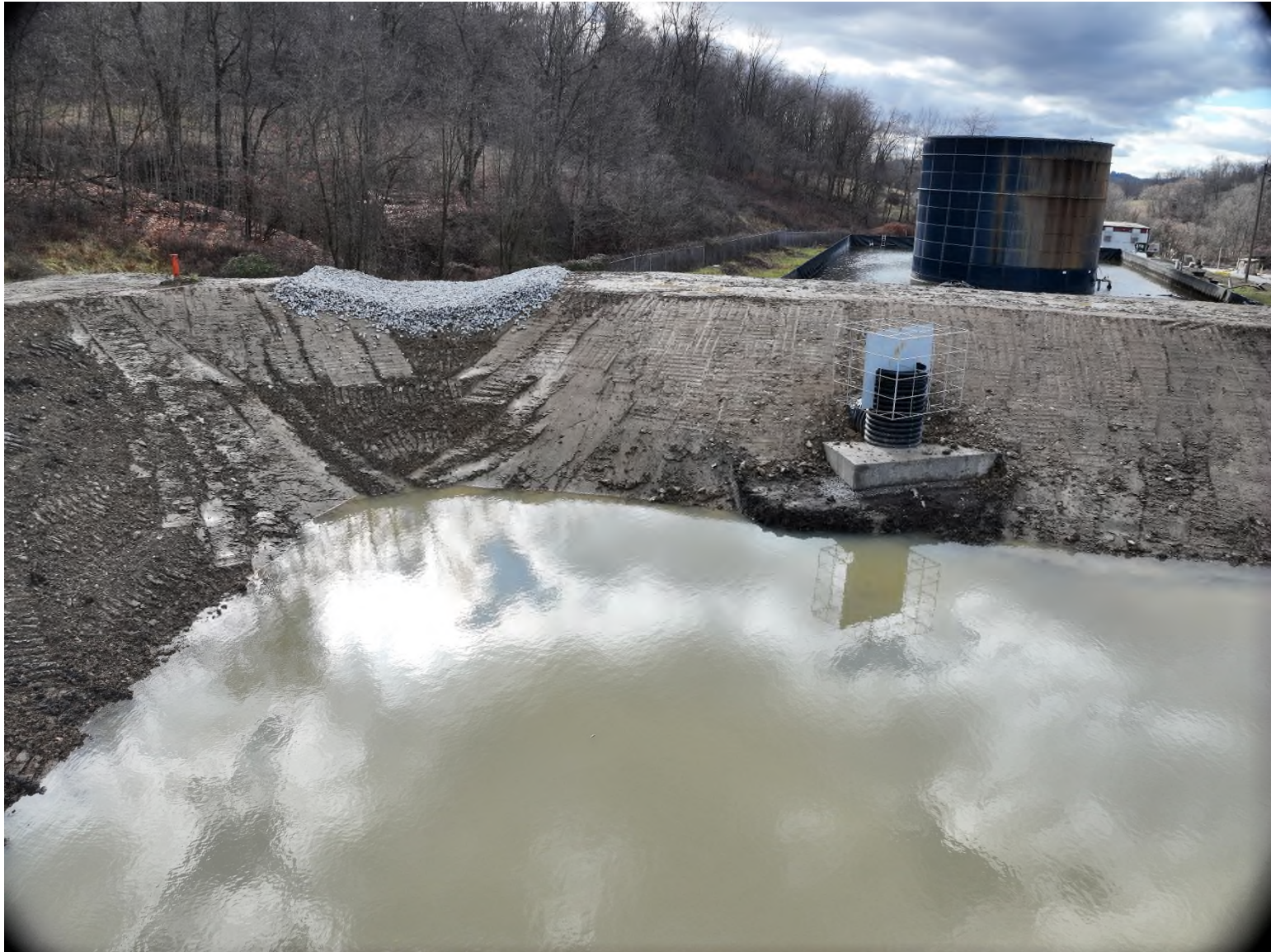
Photo 4 – Looking South at Pond C showing new riser equipped with trash rack and emergency spillway.
