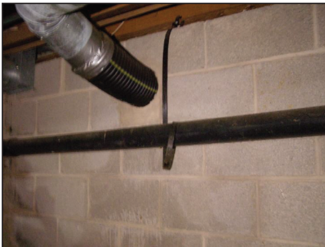
Photo #4 Broken Septic Pipe Hangars in Basement of Residence 9/17/2026 @ 13:45
