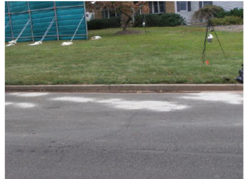
Oil dry applied to where hydraulic oil had leaked from the drilling vehicles 9-17-25 @ 13:27
