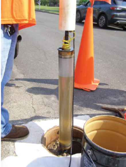
Removed skimmer from recovery well RW-2 on Glenwood Drive 8-7-25 @ 10:21am
