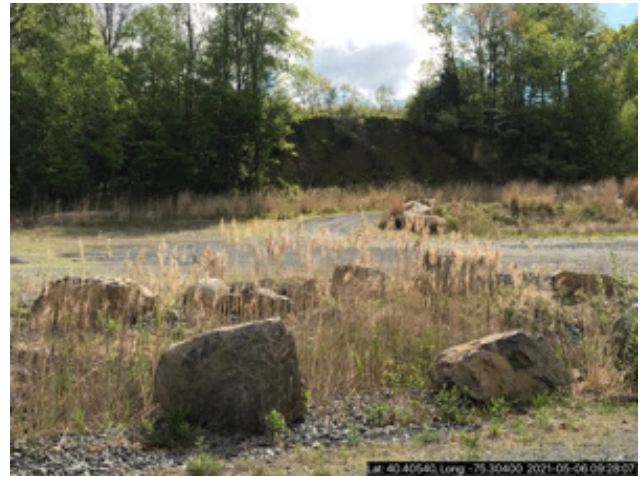
Slope near garage: vegetation growing
