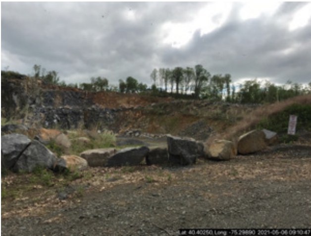
Some vegetation on S wall
