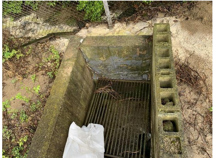
Separator and re-infiltration into the soil.
