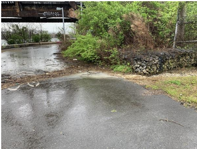
Discoloration outside of the fence line at the River Trail
