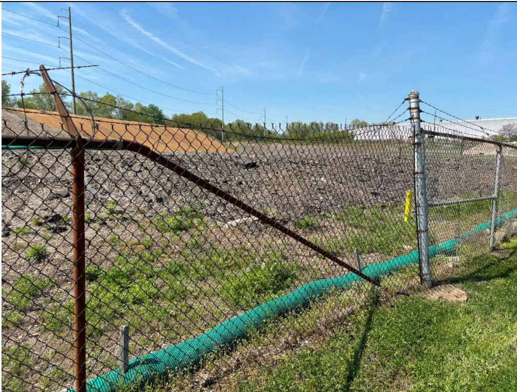
Damaged section of security fence along 51 st St. End of photo log.
