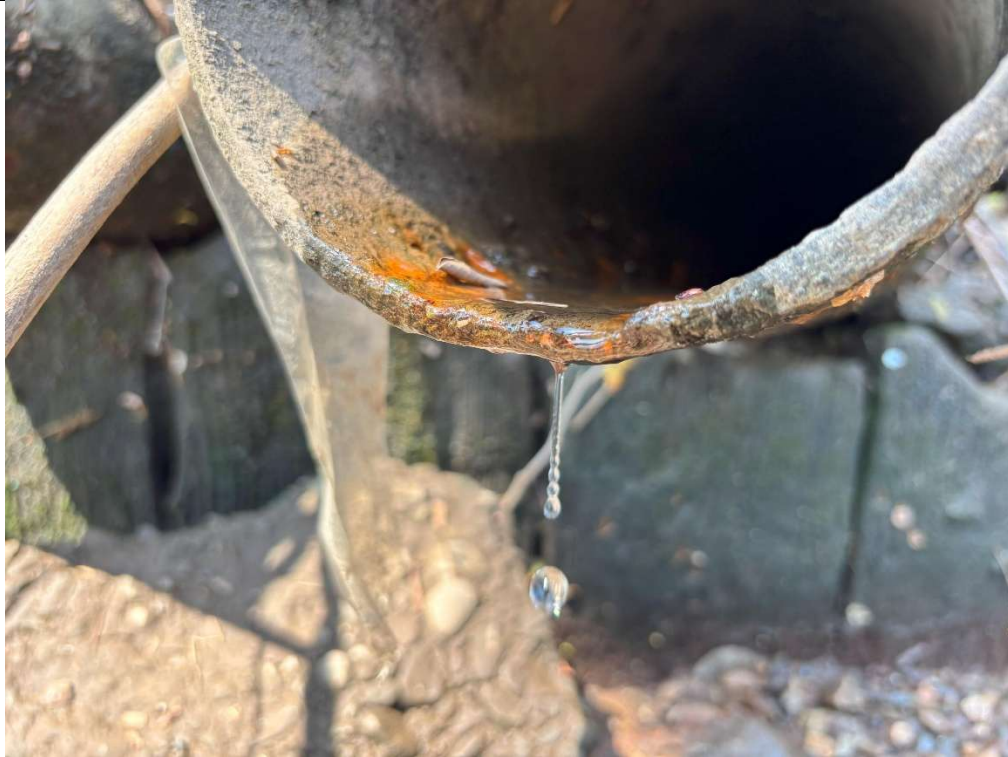
Upstream pipe outlet with drip present.
