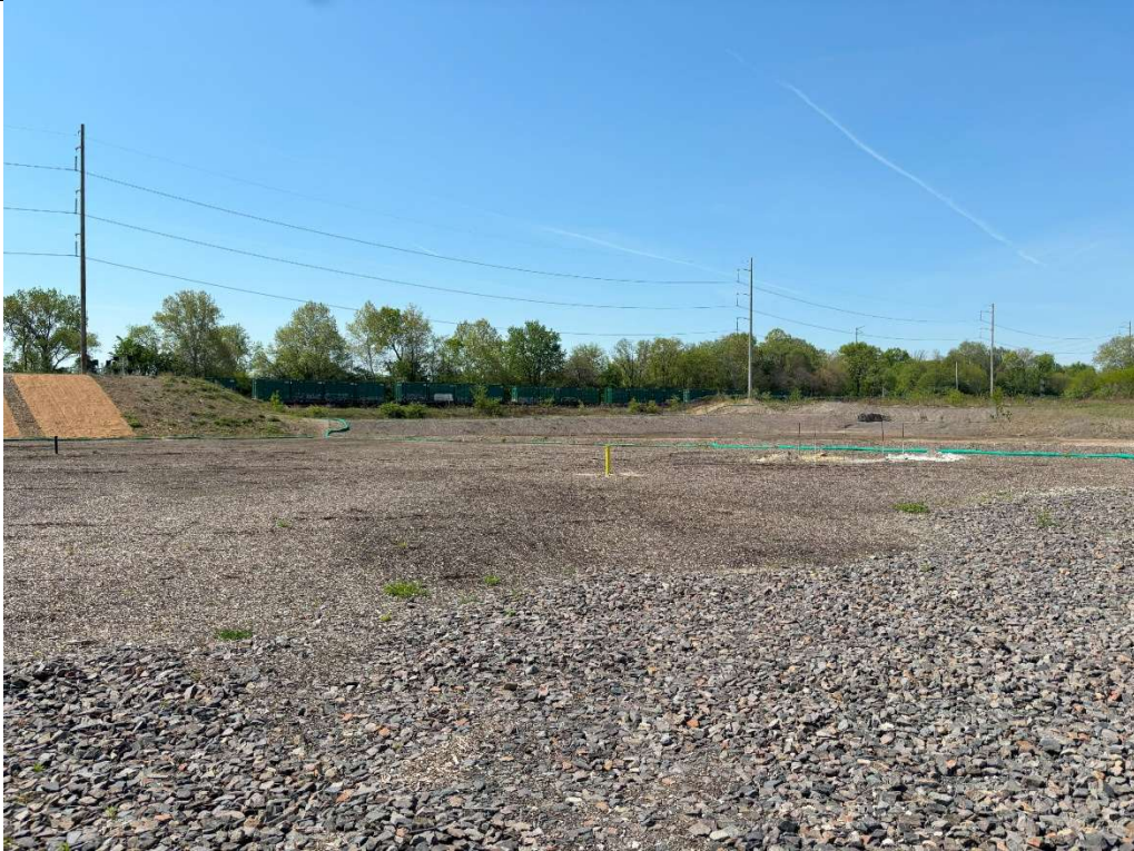
Midslope rock / rock construction entrance and mulching level of midslope portion of site.
