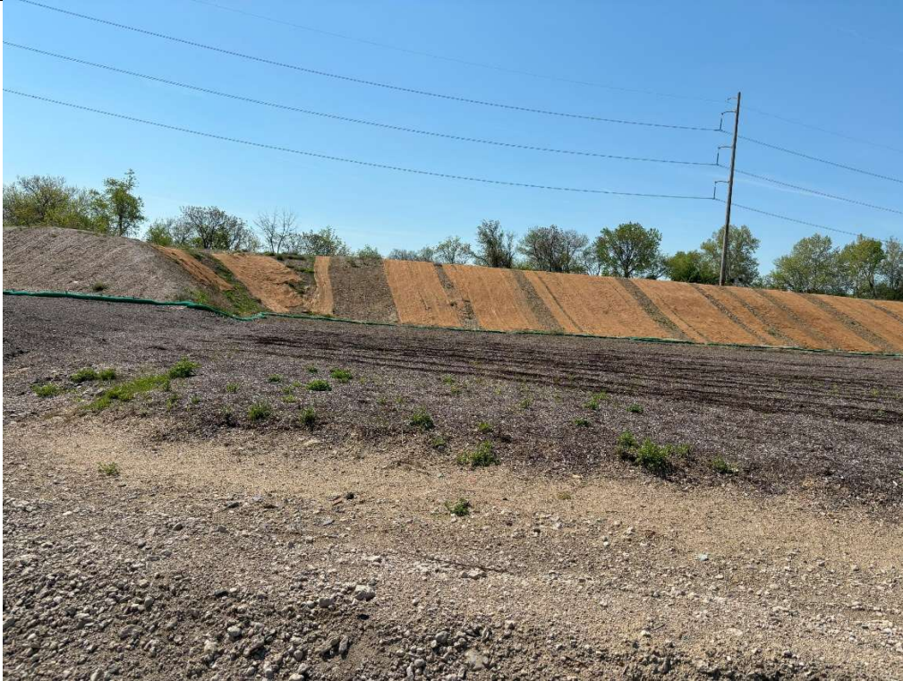
Downslope mulching levels and new erosion matting on large fill dirt stockpile.
