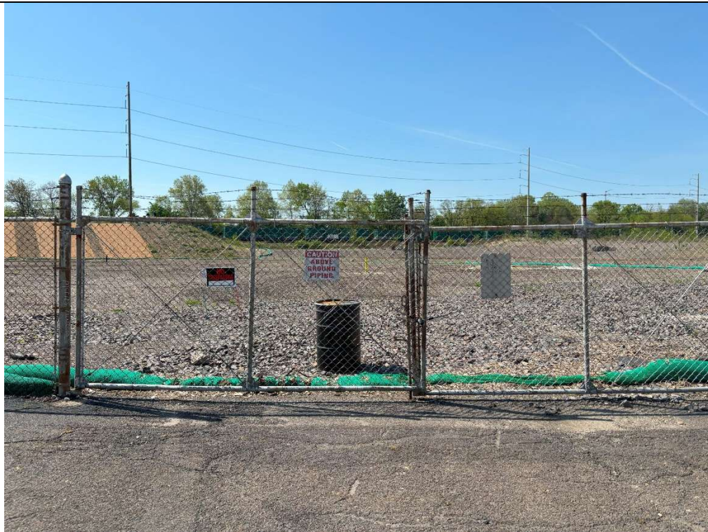
Midslope gate and damaged / run over filter sock.
