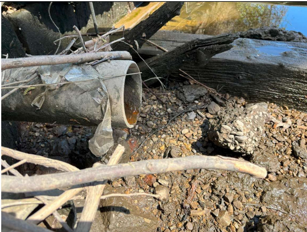
Upstream pipe outlet with drip present.
