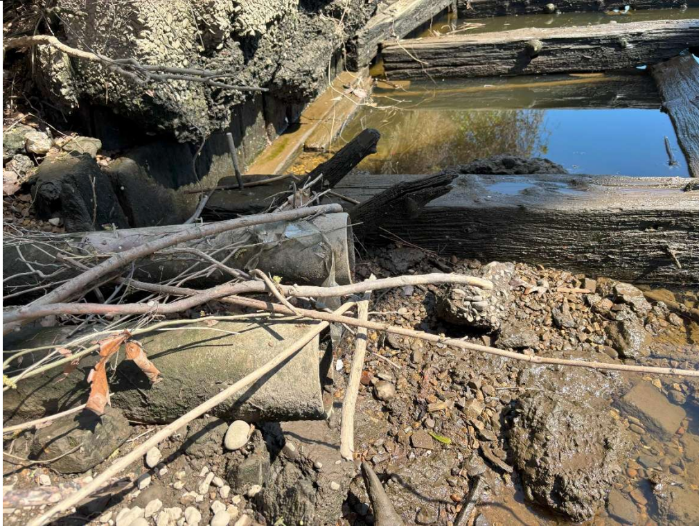
River outlet of pipes of undetermined origin at Schuylkill River across Bartram's Garden trail from site.
