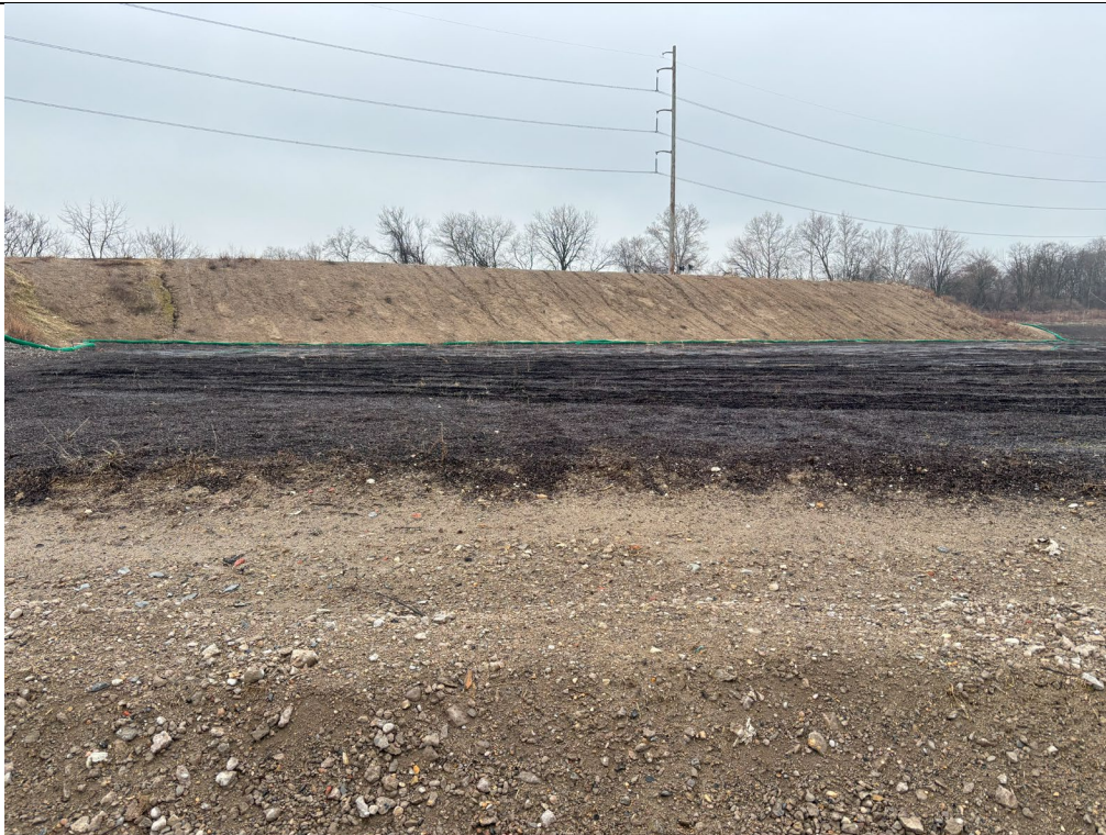
Mulched middle portion of site with large fill dirt stockpile with erosion rills and gullies present.
