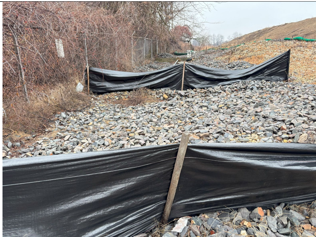
Rock lined swale and silt fence.
