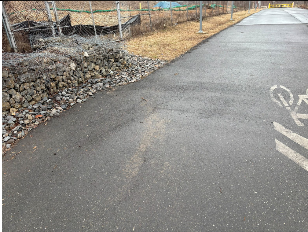
Site of previous sediment staining on Bartram's Garden trail.
