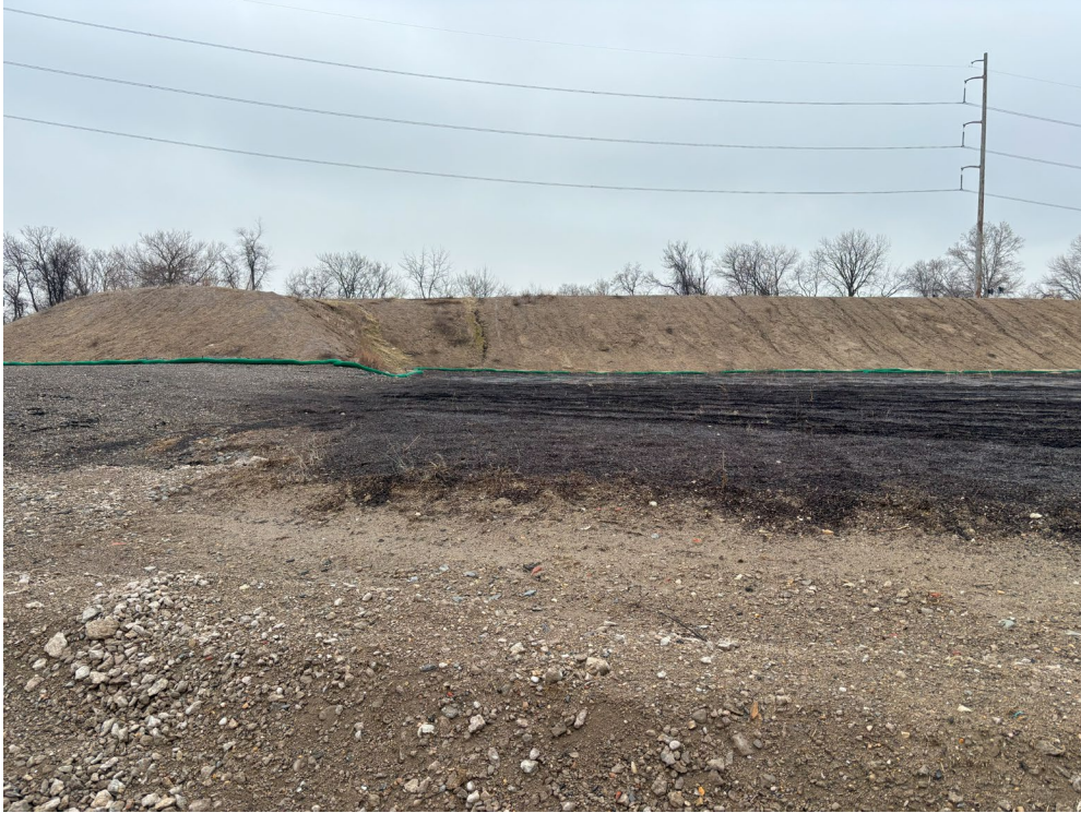
Mulched middle and lower portion of site with large fill dirt stockpile indicating erosion rills and gullies.
