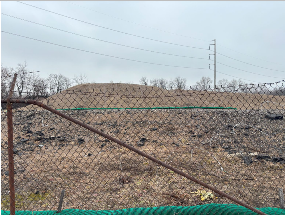
Damage to perimeter fence and concertina wire.
