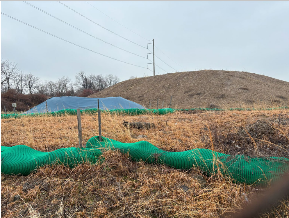
Downslope end of large fill dirt stockpile, small contaminated fill dirt stockpile covered in blue tarp, and downslope filter sock.
