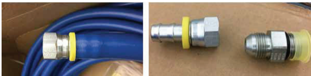
Figure 3.17 – Compressed Air Line Connection to the Dosing Cabinet
