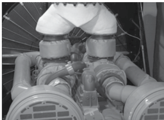
Figure 3.9 – Exhaust Piping Insulation
