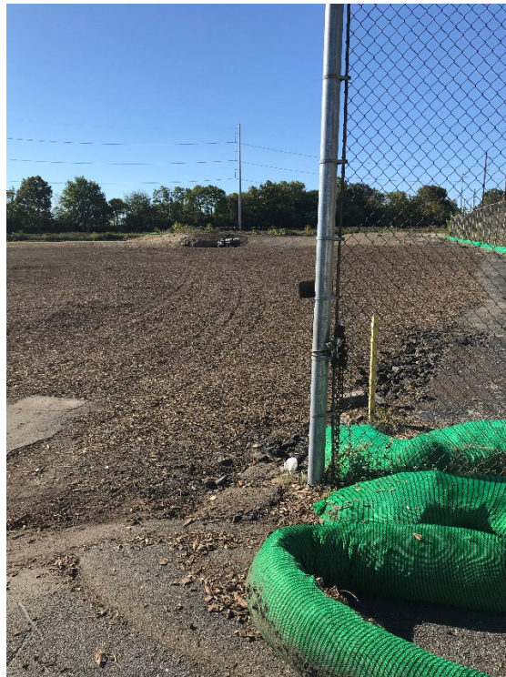
Upslope portion of site with soil matting (E&S) work being done in distance.
