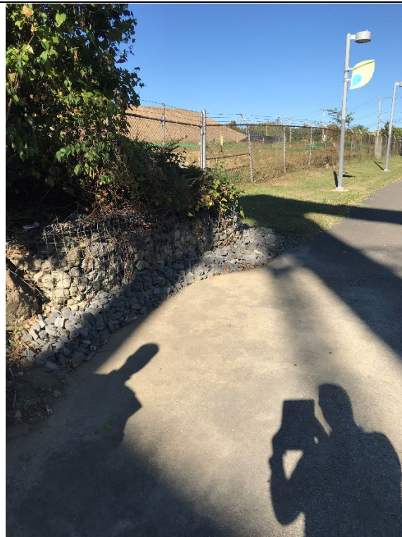
Sediment staining on Bartram's Garden trail.
