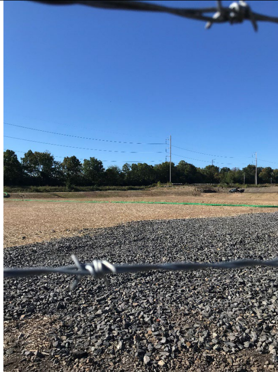
Middle portion of site, looking upslope, with soil matting (E&S) work being done in distance.
