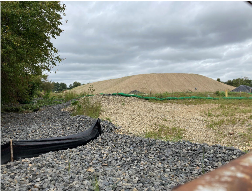
Large fill dirt stockpile with small amount of germination through mulch and matting present, looking from Bartram's Trail.
