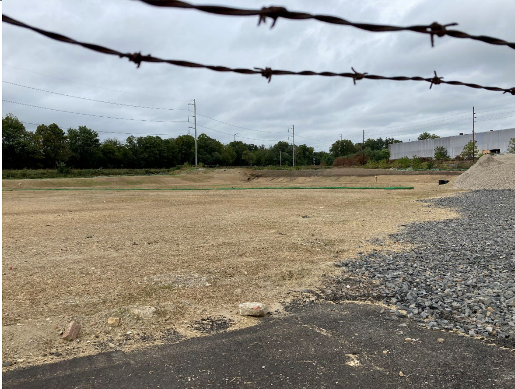
Mulching of middle and upslope portions of site, looking from 51 st St.
