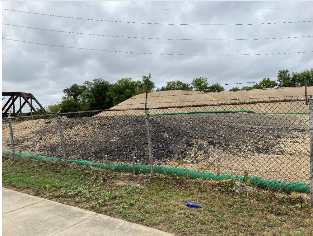
Asphalt millings in foreground and stabilized large fill dirt stockpile in distance.
