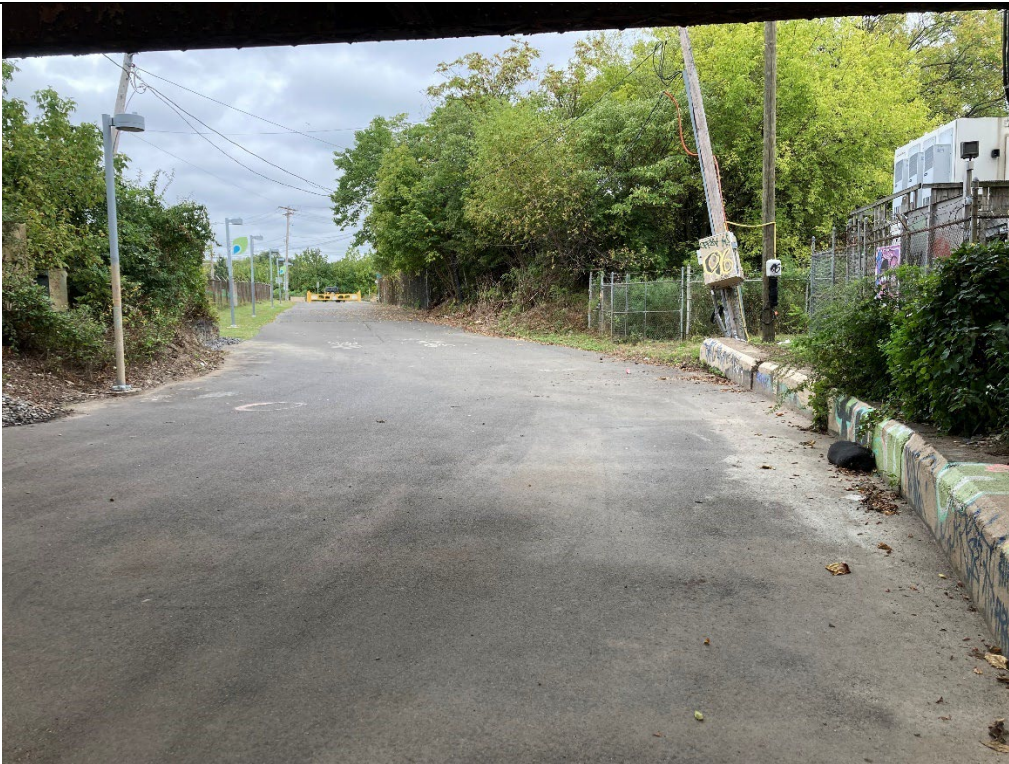
Sediment staining on Bartram's Garden trail.
