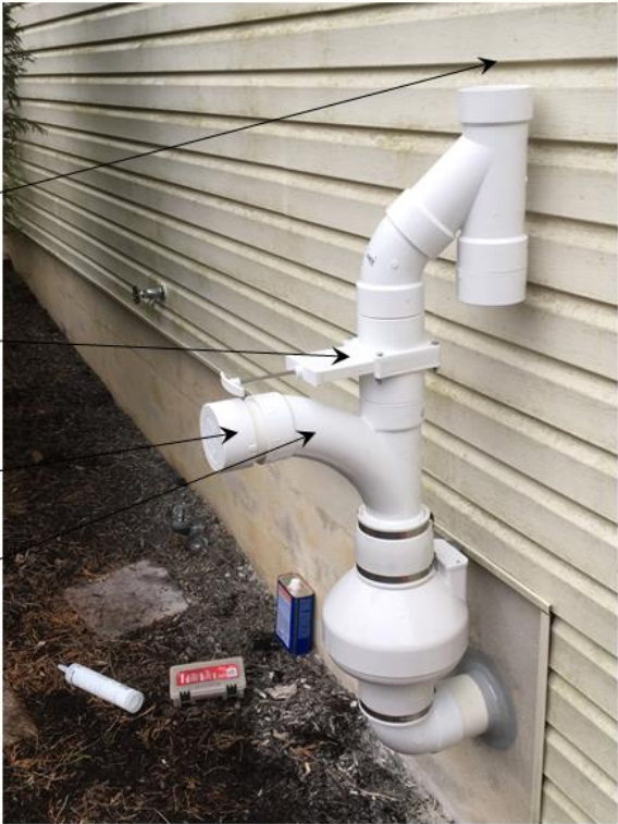
Photo 1. Reconfigurable mitigation system apparatus installed at all study houses allowing for changing between roofline and ground level exhaust configurations.
