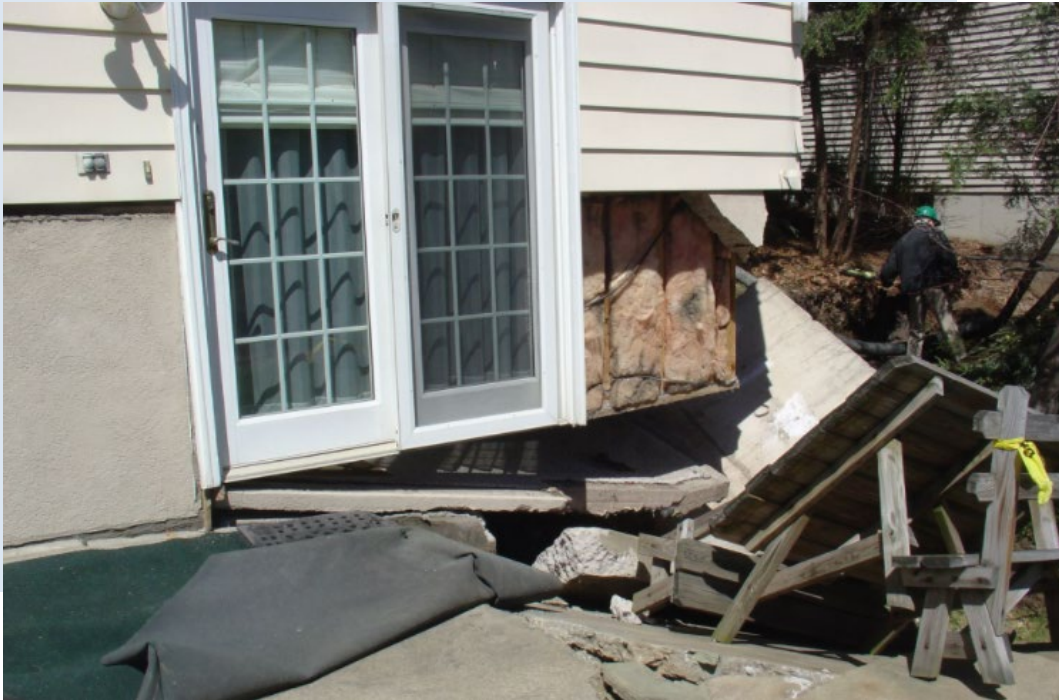
Figure 2. Example of a structure in Pennsylvania damaged by mine subsidence.
