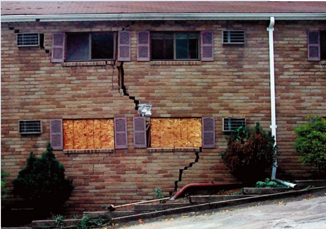
Figure 1. Example of a structure in Pennsylvania damaged by mine subsidence.
