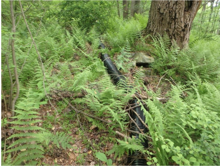
Figure 2. Perennial watercourse 041017_GM_1001_P_MI flows through approximately 275 feet of 8-inch diameter flexible pipe culvert on the north side of the access road. (View facing north)
