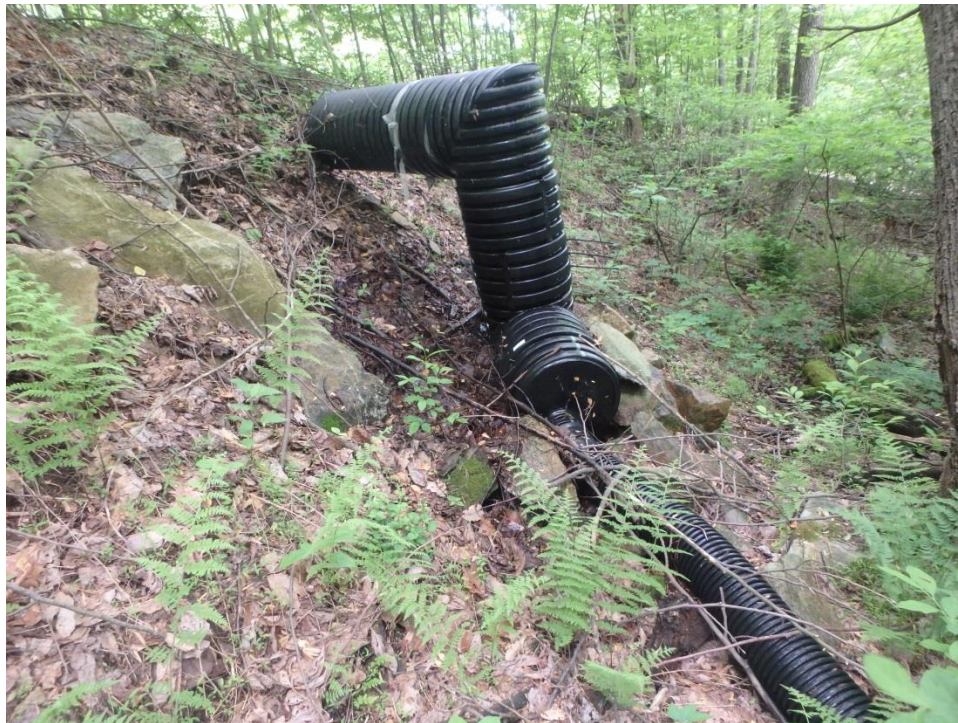
Figure 1. Perennial watercourse 041017_GM_1001_P_MI flows through a culvert under an existing dirt/gravel access road. (View facing southwest)
