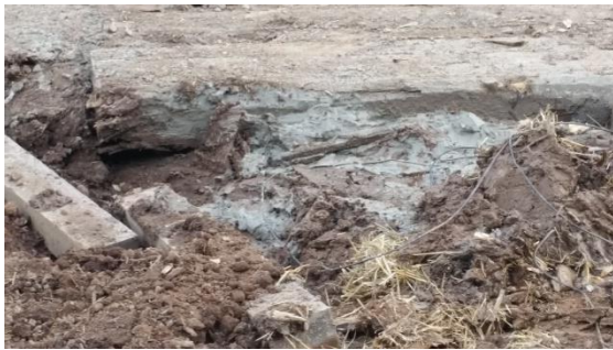
Inadvertent return of drilling fluids (grey)
