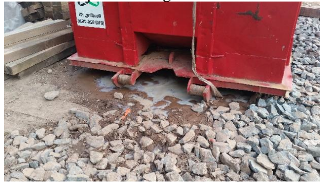
Roll off dumpster leaking some unknown fluid
