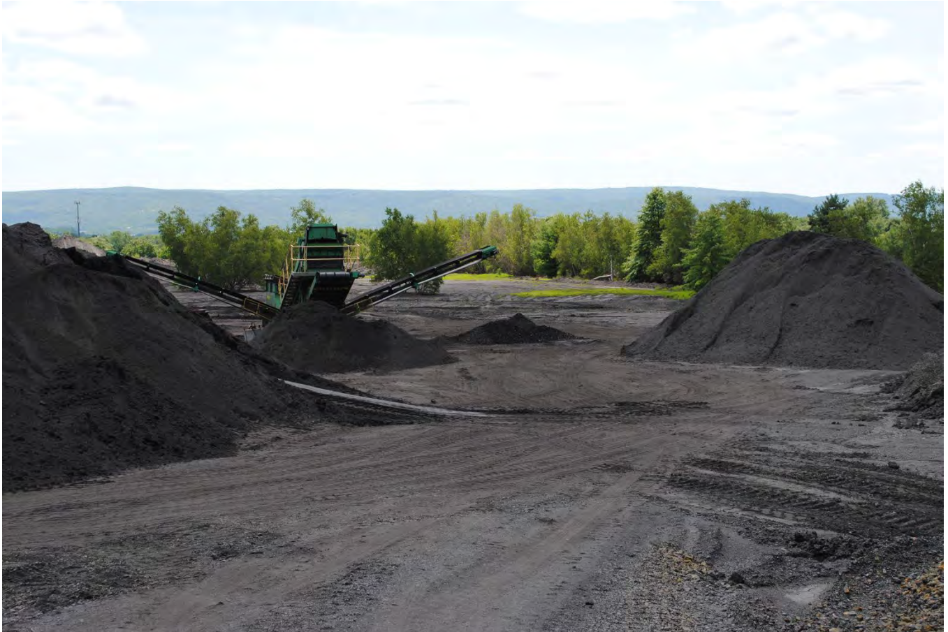
Material Processor moved up onto the upper basin level looking South, Date: 7/15/19
