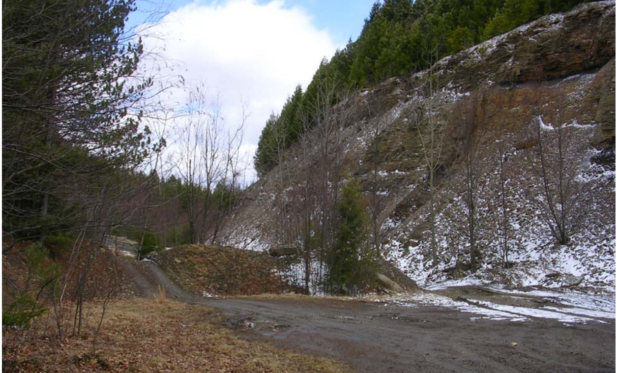
Figure 15. High-priority unreclaimed dangerous highwall located on State Game Lands in the Bennett Branch Watershed.
