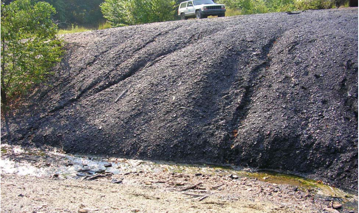
Figure 22. Refuse pile cast along Tyler Reservoir Run south of the Village of Hollywood in Huston Township, Clearfield County.
