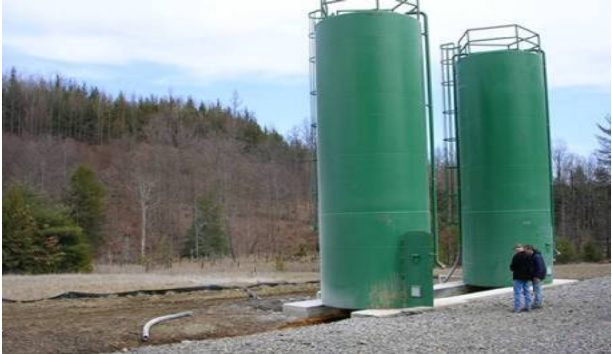
Figure 20. Lime silos for a tipping bucket lime doser treating another mine discharge in the Porcupine Hollow Tributary of Dents Run.
