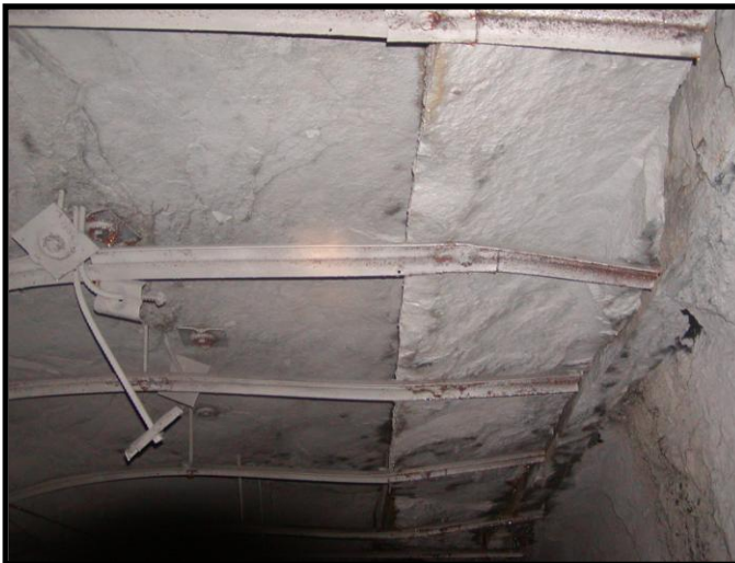
Underground Roof Crack
