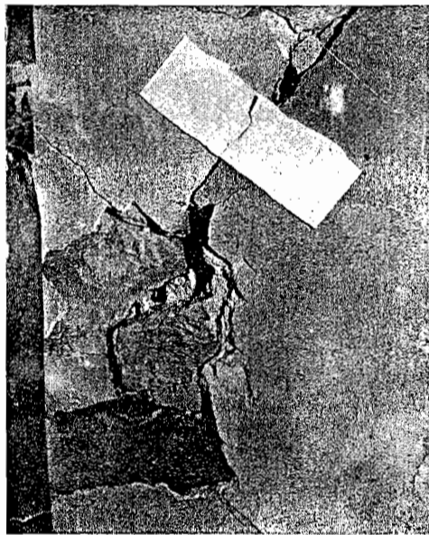
Fig. 5—Showing tell-tale across an original crack
