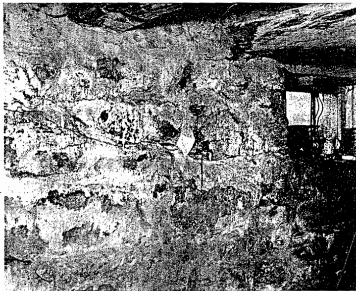
Fig. 9—Horizontal crack—building F
