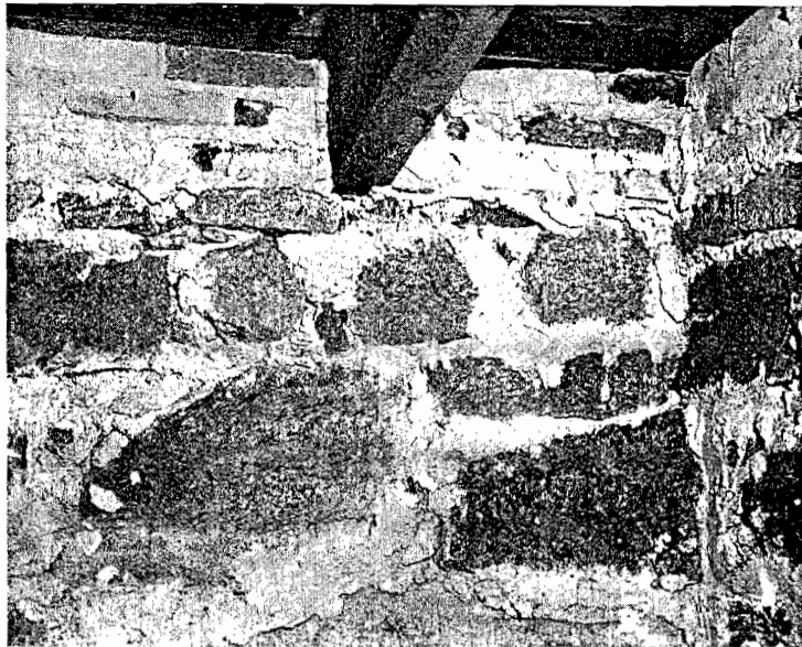
Fig. 8—Horizontal crack—building T
