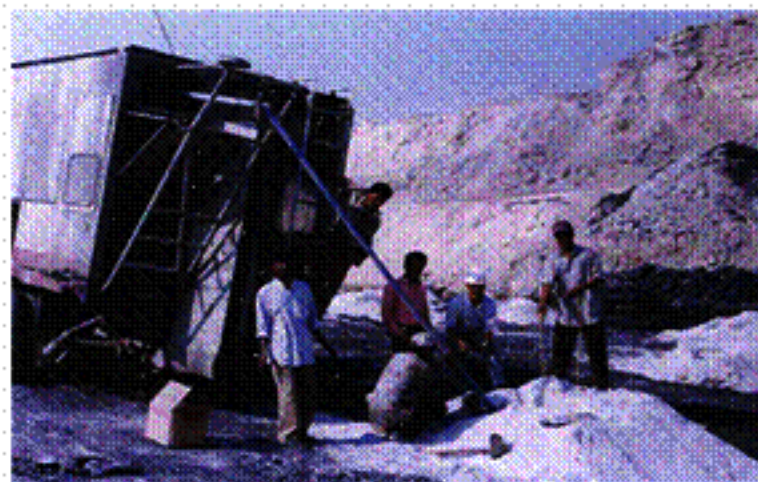
Figure 3.5 Field photographs showing lowering of probe cable and EXEL initiation system (top) and charging with SMS explosives (bottom)
