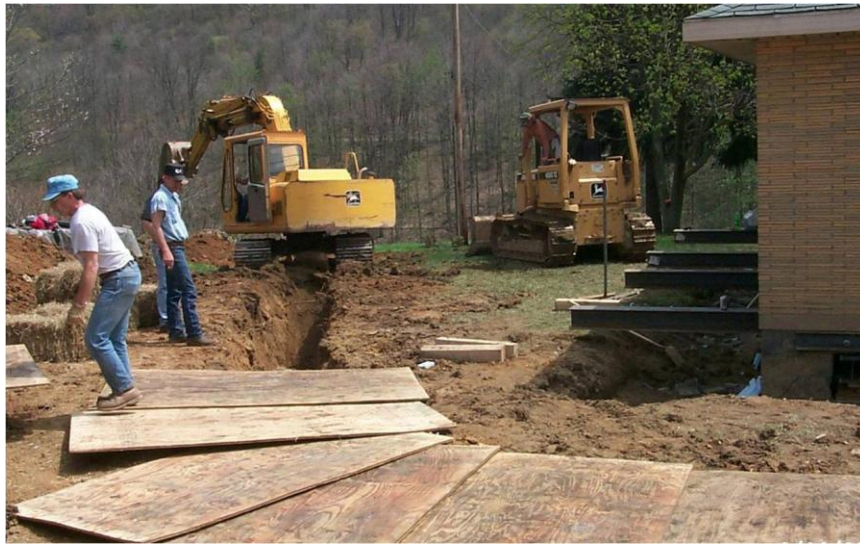
Figure V-16 - Photograph of a trench excavated adjacent to a structure to mitigate high horizontal strains (Photograph from PA DEP files).
