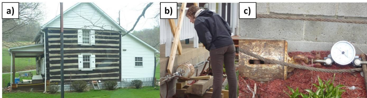
Figure V-13 - Photographs of a) residential structure with polypropylene rope around the foundation, b) steel cable spring and tension assembly, and c) spring and gage assembly (photographs courtesy of N. Iannacchione).
