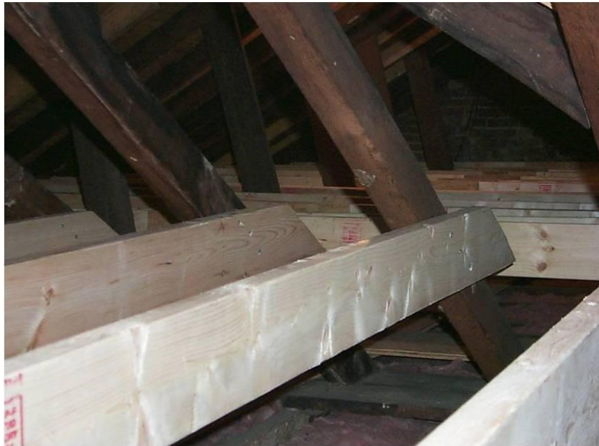
Figure V-15 - Bridging applied to a structures attic to stabilize the roof (Photograph from PA DEP files).
