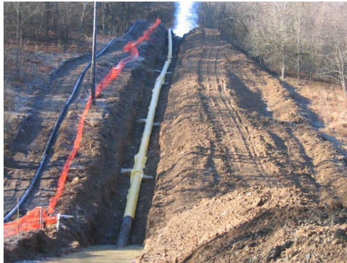
Figure I-10 - Gas pipelines are routinely excavated and temporarily supported to mitigate the impacts from longwall mining (Photograph from PA DEP files).
