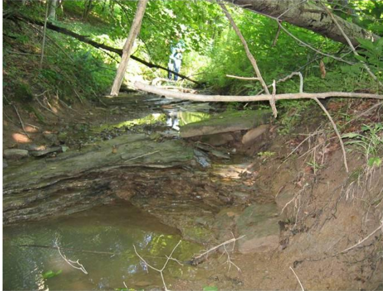
Figure D-7 - Small compression ridge observed in the 3N panel post-mining (Photograph from PA DEP files).
