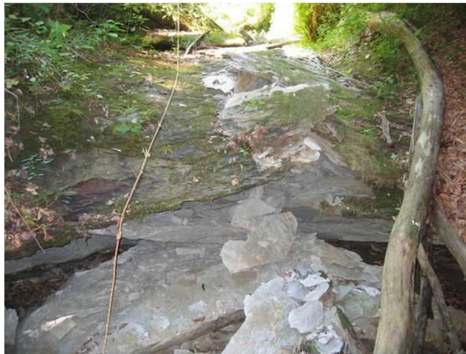
Figure D-1 - Compression ruptures observed by PA DEP during post-mining survey of the 7H panel in Bailey Mine (Photograph from PA DEP files).
