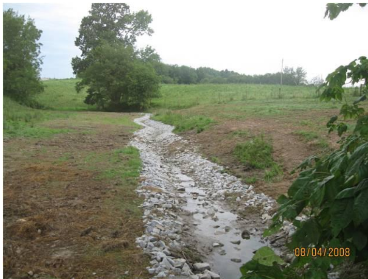
Figure D-11 - Mitigation work observed by PA DEP during a post-mining survey (Photograph from PA DEP files).
