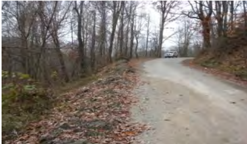
Unstable Road Slide Area
