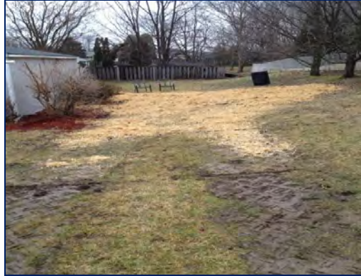
Bulls Head Road Subsidence
