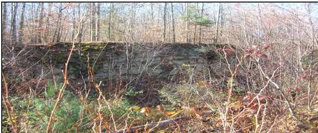
Dangerous Highwall Area
