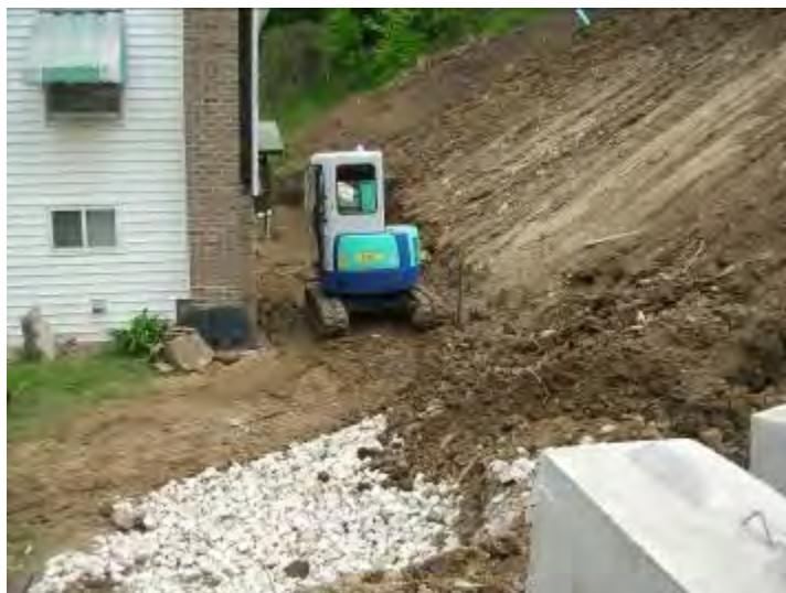
Removal of the slide material with no damage to the main structure and re-establishment of a stable slope was accomplished quickly.
