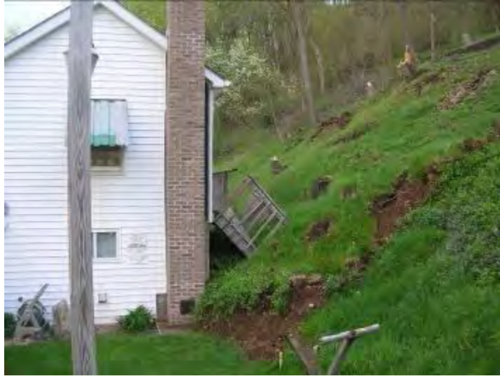
Approximately three feet (3') of saturated ground slid against the back of the house and collapsed the second floor deck.
