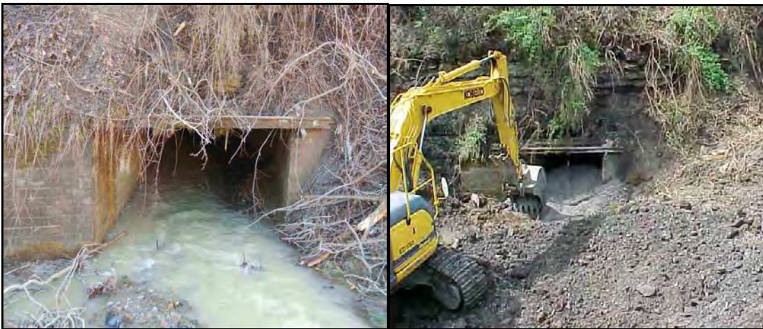
Maude Mine opening before (left) showing Fishing Run stream flowing uncontrolled into the entry and sealing of the opening (right) during reclamation
