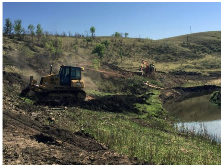
Lovejoy Avoca Coal Fire Emergency, June 3, 2015: Earthworm Excavating was uncovering burning coal fines with a Cat D-6 bulldozer and excavating a burial trench with a Cat 316 Excavator for the burning materials. Note the sinkholes in the background.
