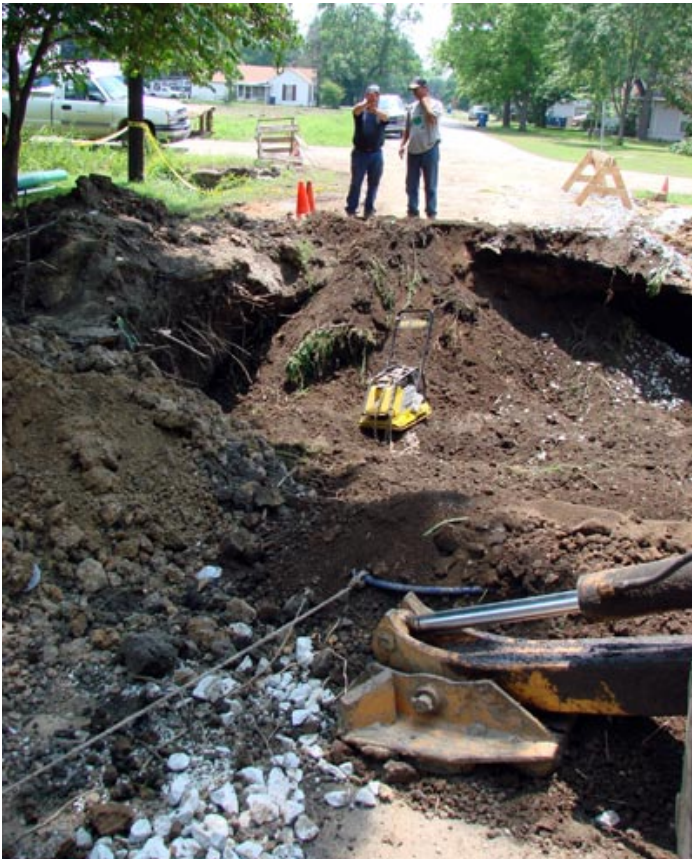
Arno Street Sinkhole
