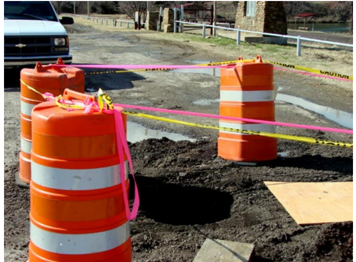
McCurtain Park Sinkhole
