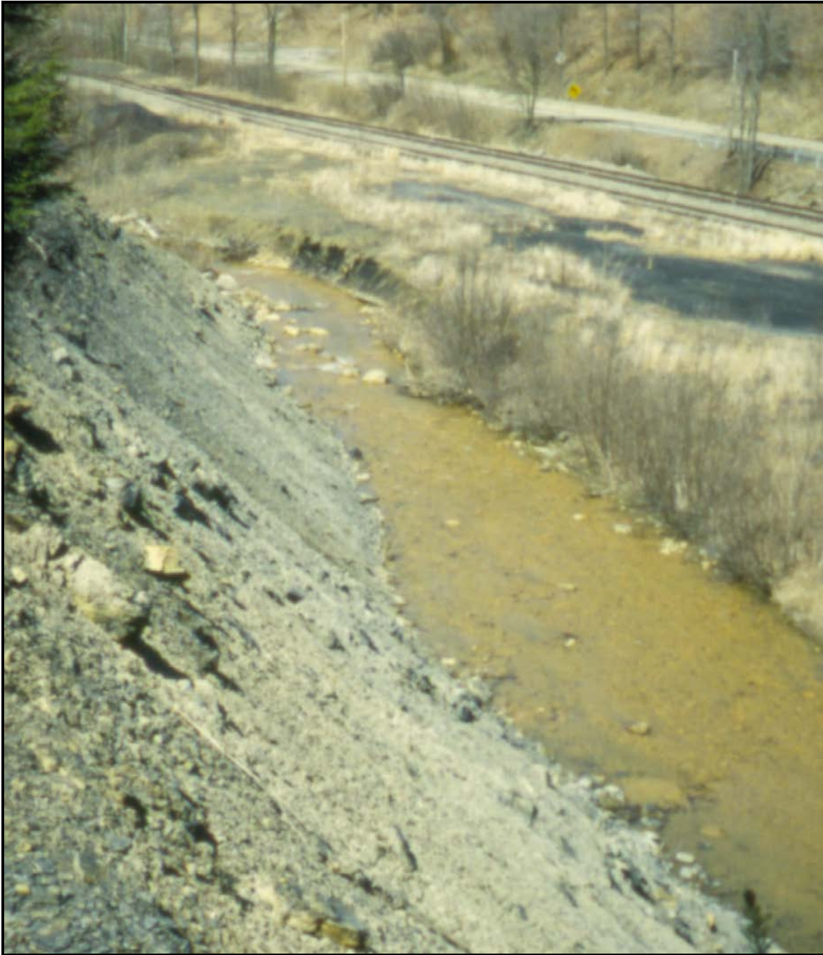
FIGURE 4 – Photograph showing the extremely steep outslope of the coal refuse pile with the toe of the pile extending into the stream channel. The iron stained stream bottom of Sugar Creek is also evident in the photograph.
