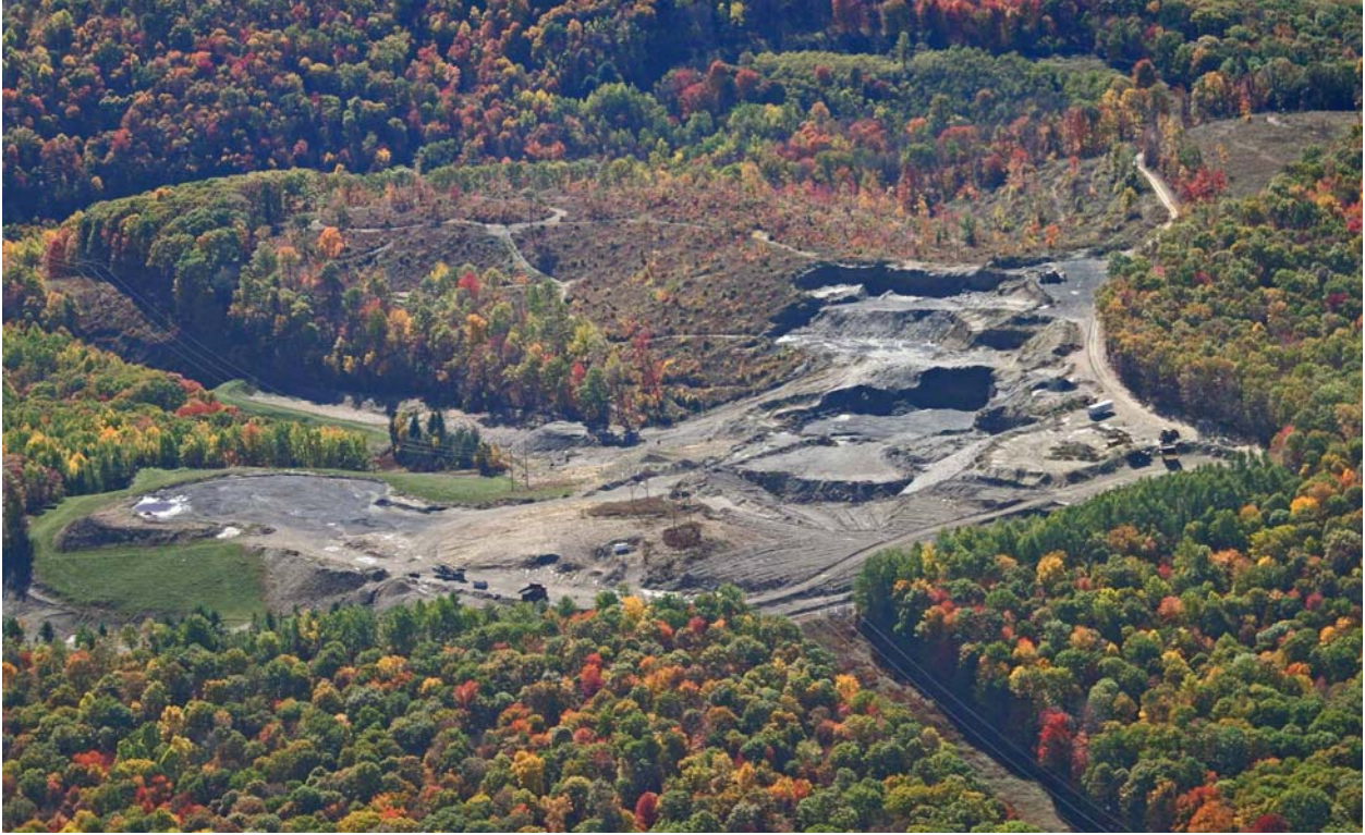
Figure 24. Amfire Mining Company surface mine in the Mill Run Tributary to Bennett Branch in Huston Township, Clearfield County.
