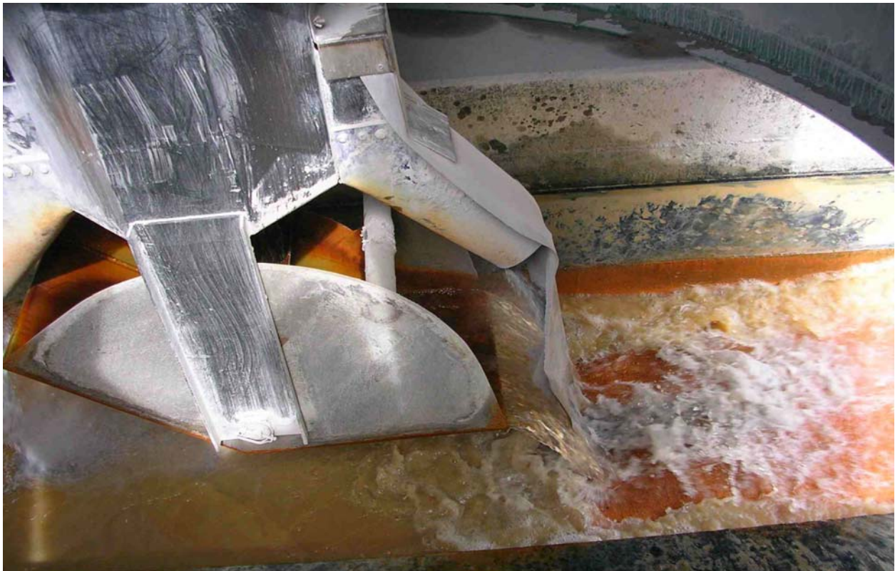
Figure 21. Tipping bucket mechanism dispensing lime to neutralize the highly acidic discharge.
