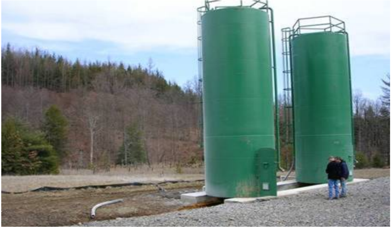
Figure 20. Lime silos for a tipping bucket lime doser treating another mine discharge in the Porcupine Hollow Tributary of Dents Run.
