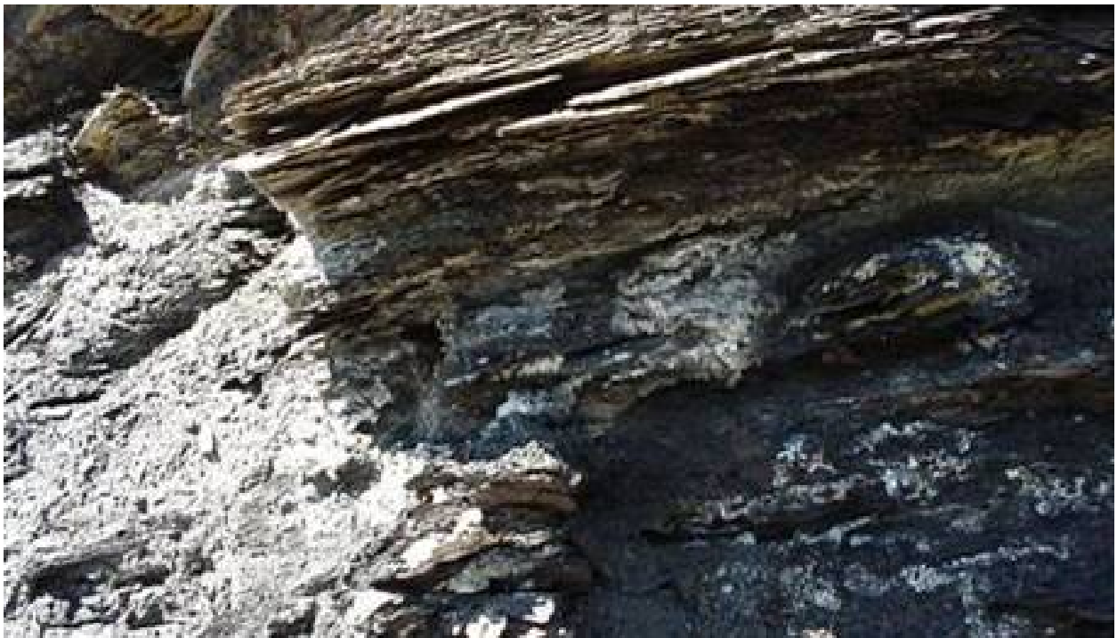
Figure 16. Sulfate salts crystallized on the rocks of an unreclaimed dangerous highwall located on State Game Lands No. 311 in the Bennett Branch Watershed.
