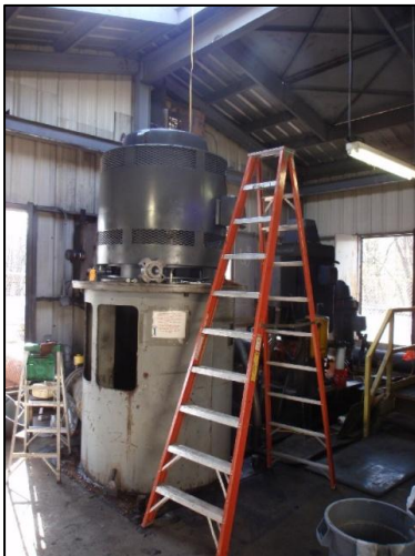
State-operated pump at Gilberton, Schuylkill County, one of the remaining MWCP pumps in operation. This pump is currently operated to protect several hundred homes in Gilberton Borough whose basements and foundations are below the overflow level of the minepool - M. C. Korb, 2010
