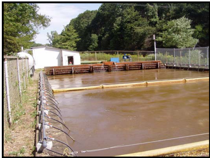
Figure Lasaire-11. Lasaire Aeration System at the Wildwood Treatment System.
