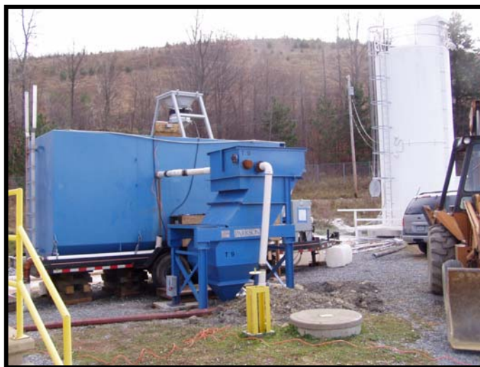
Figure Brandycamp-4. Pilot System Setup at the Brandycamp AMD Treatment System
