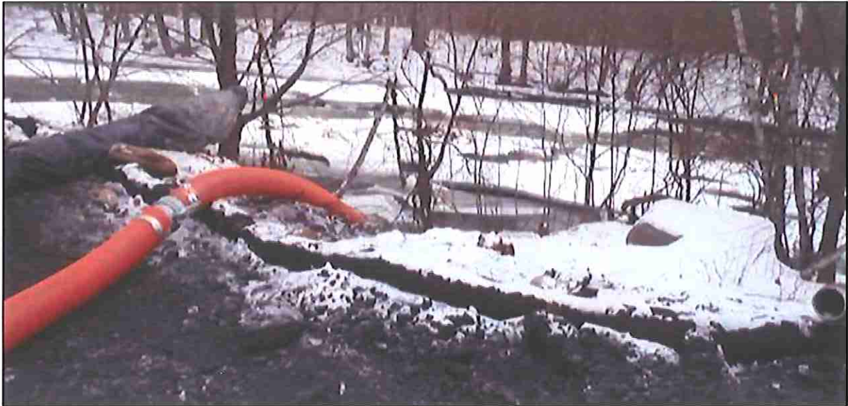
Pump Suction in 32°F Lackawanna River January 2014 – PADEP BAMR
