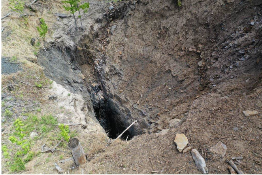
AMLF 0435-18 (VO): Looking Southeast at the vertical opening and subsidence with underground mine workings visible, depth to mining is approximately 189 feet.
