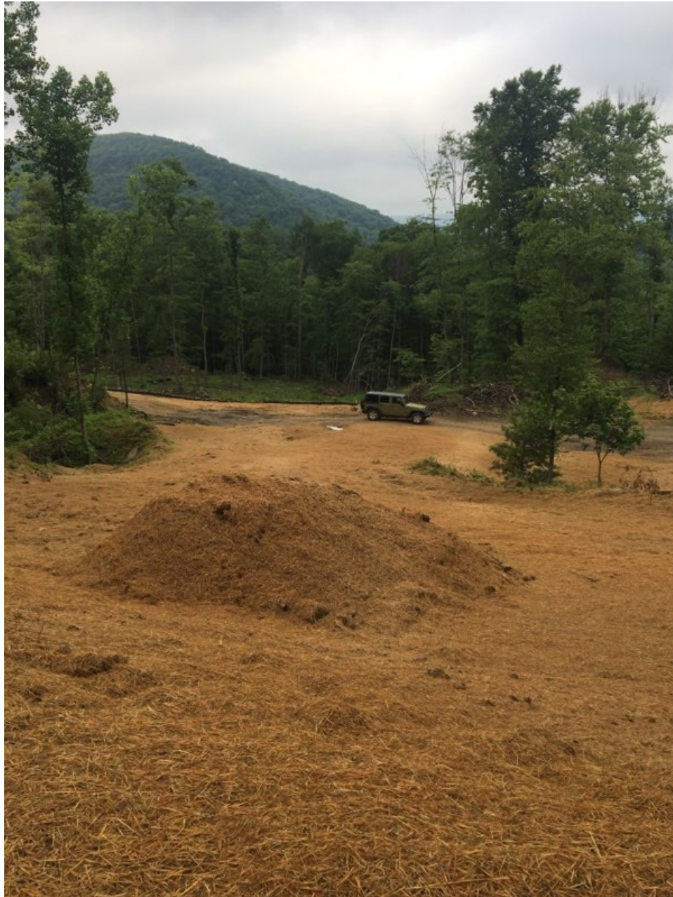
Looking North, vertical opening feature is reclaimed, filled completely with mine refuse, and a six (6)-foot mound placed atop the feature. Project area seeded for revegetation.
