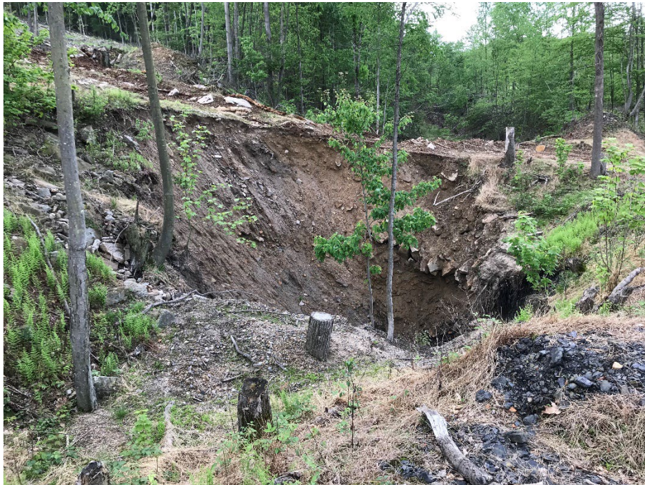
AMLF 0435-18 (VO): Looking East, this vertical opening is 40 feet in diameter at the surface, 10 feet in diameter at the bottom, and 40 feet deep.
