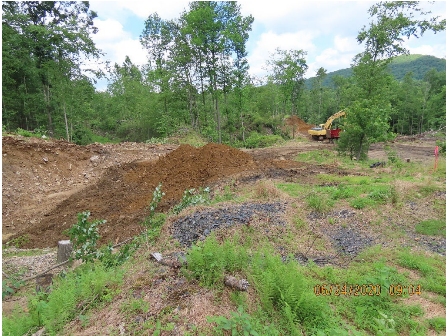
Backfill of subsidence in progress: looking Northwest. Excavator is removing mine refuse from designated borrow area.
