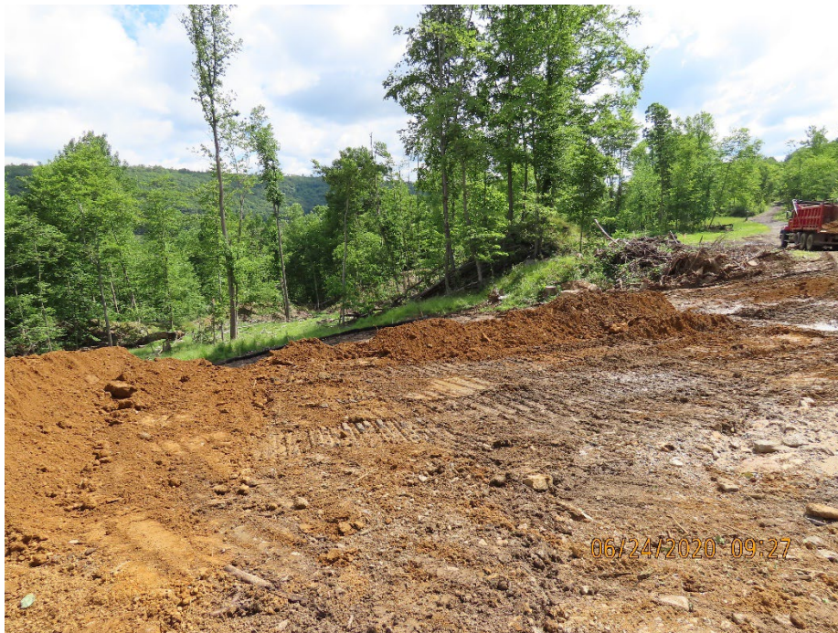
Looking Northeast, contractors utilize the ATV trail as a haul road to remove backfill from borrow area.
