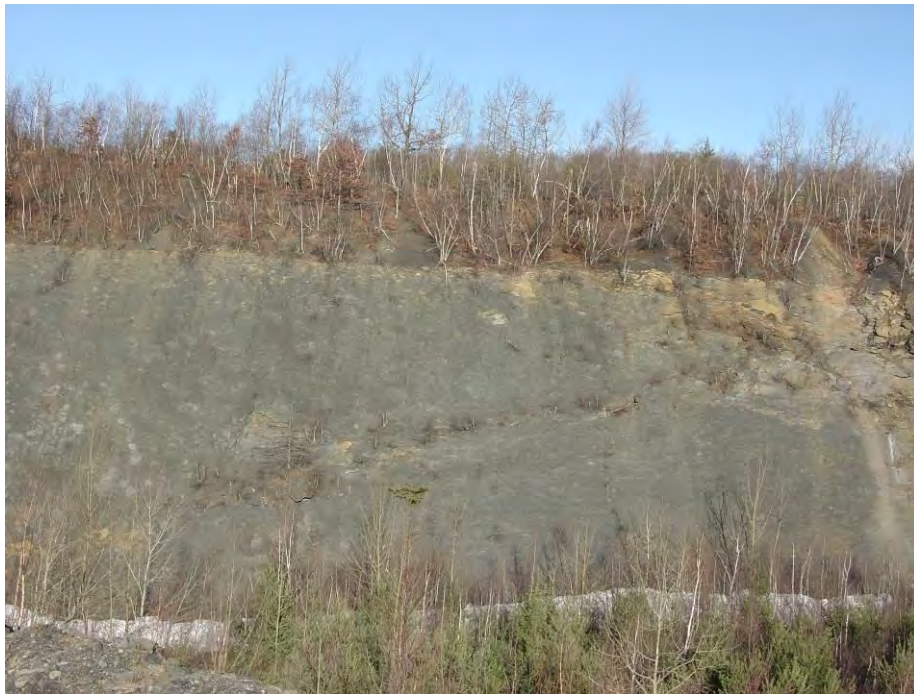
Photo of Dangerous Highwall #1 looking north at northern highwall. Part of Dangerous Pile Embankment#11 is visible on top of highwall.
