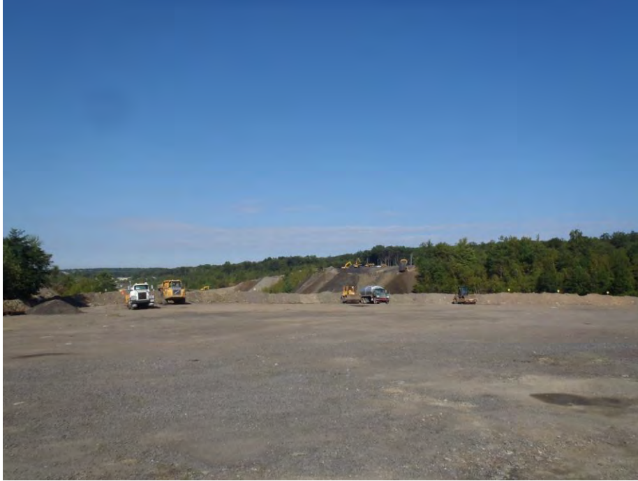
Photo of Dangerous Highwall #1 looking to west.
