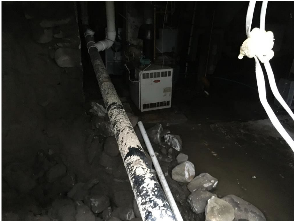
AMLF 2237-10 (VO): In the southwest corner of the basement, the subsidence appears to be choked off by foundation material and soil with no venting observed.
