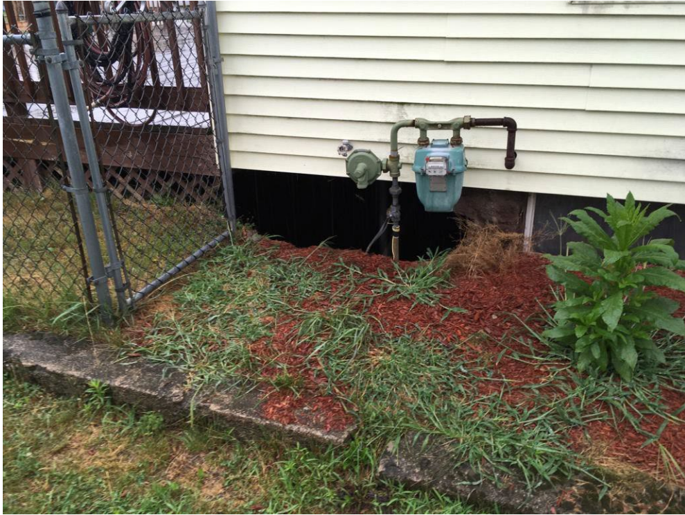
AMLF 2237-10 (VO): Looking northeast, approximately five (5) feet of the foundation wall and approximately ten (10) feet of the adjacent foundation wall collapsed into the subsidence.
