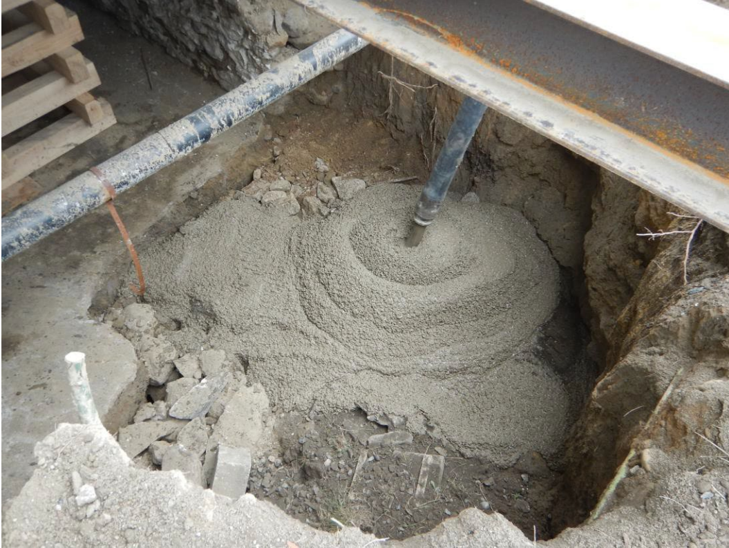
Backfilling subsidence in basement with concrete material
