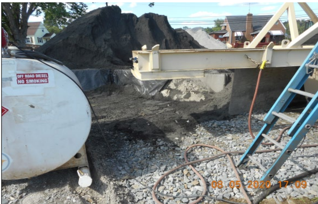
FAIRHOPE (MULTI-STRUCTURE SUBSIDENCE) CONTRACT NO. OSM 26(2757)102.1 EMER
