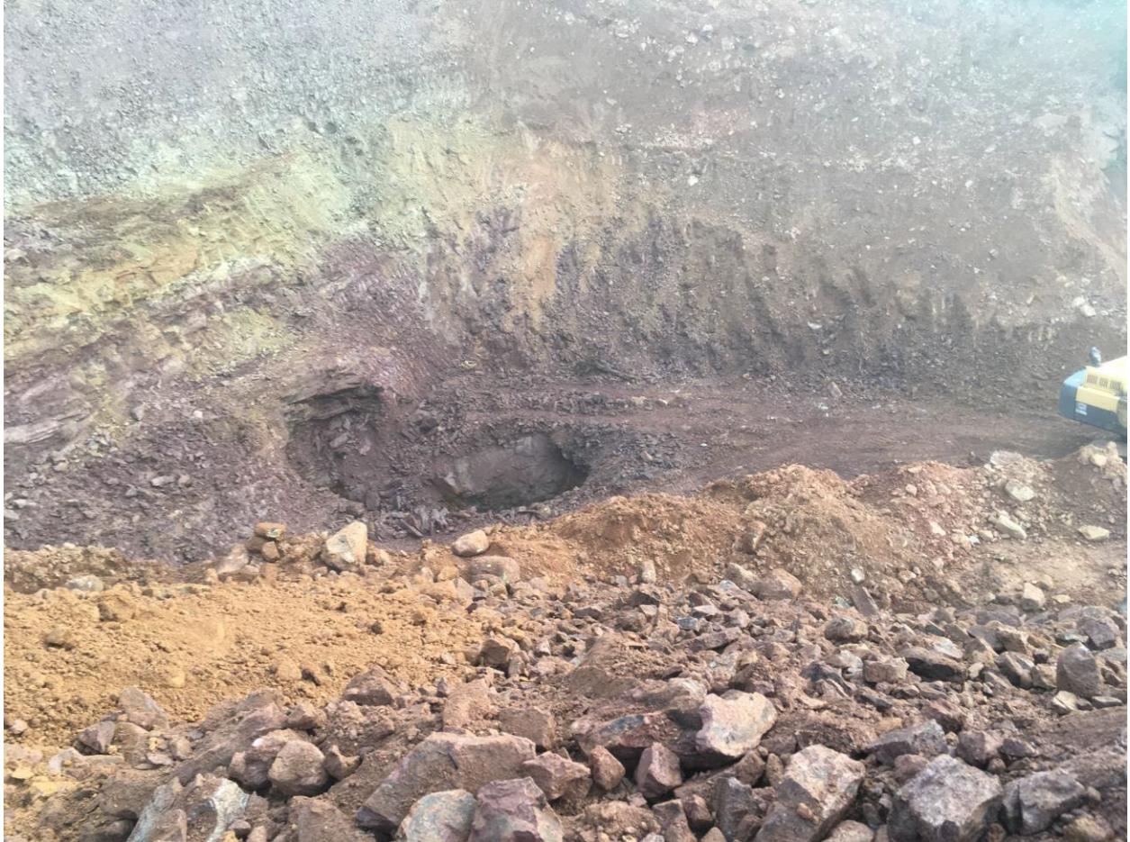
Subsidence Area Tunnel Roof Exposed
