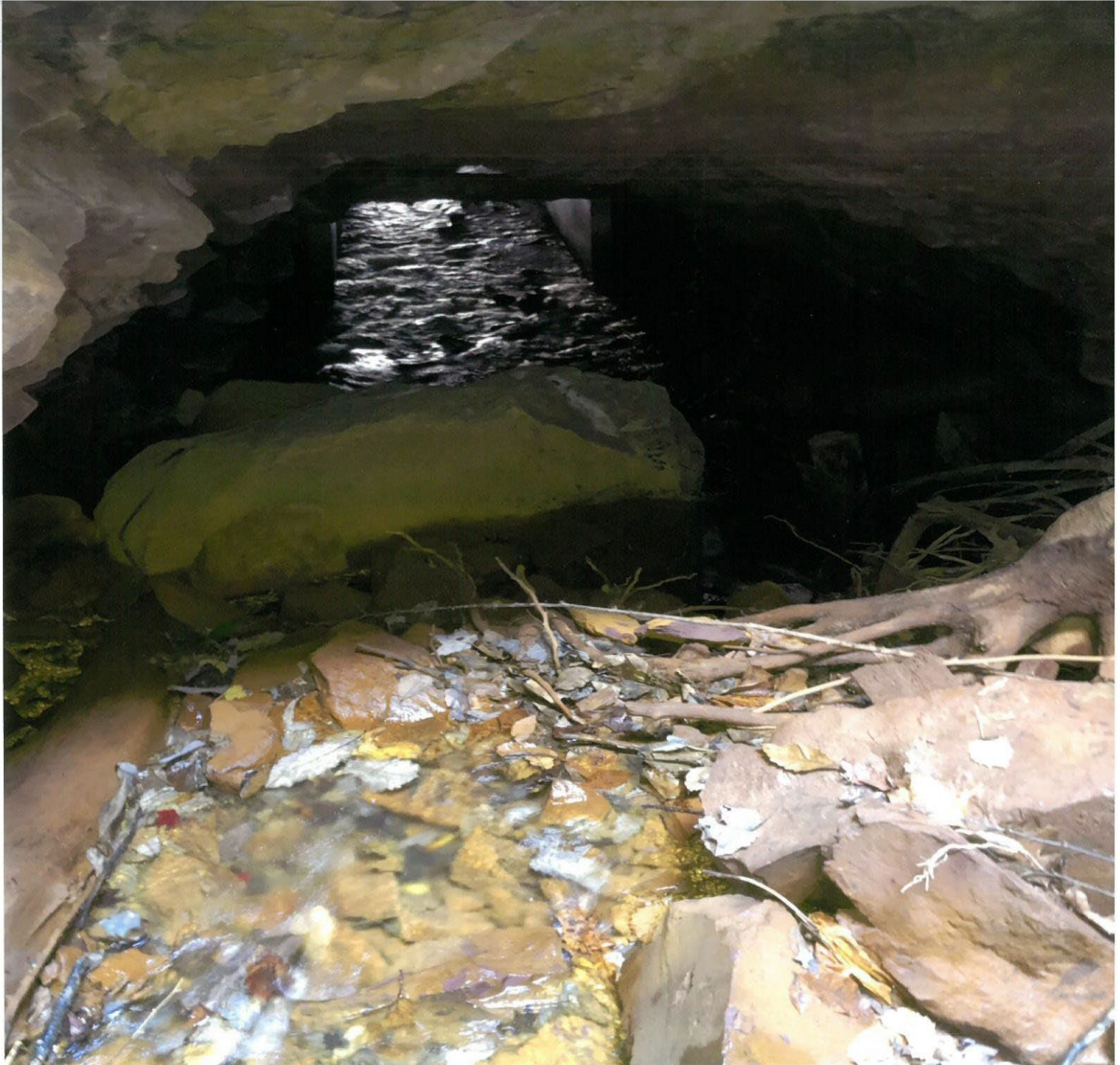
Tunnel Blockage at Subsidence Location
